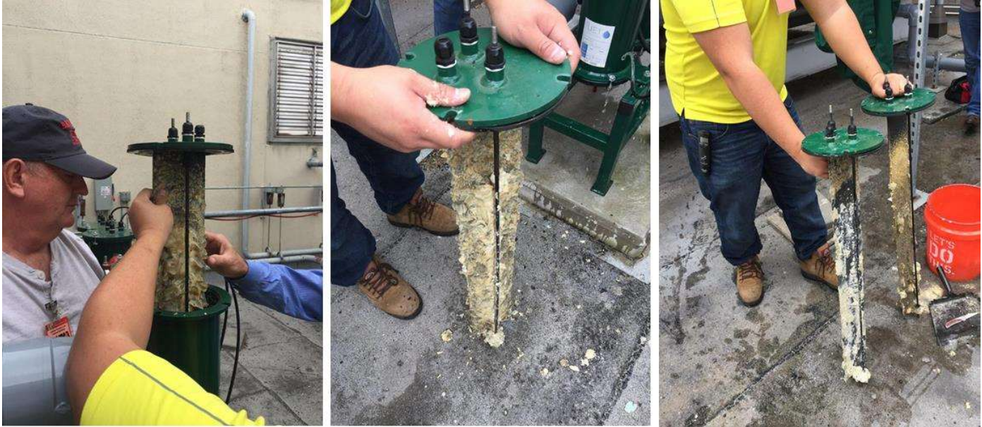
Figure 4. Cleaning the AWT System (Credit: Gregg Tomberlin, NREL)
