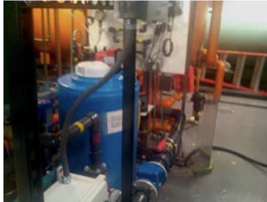
Chemical Tank – Proprietary Solution
