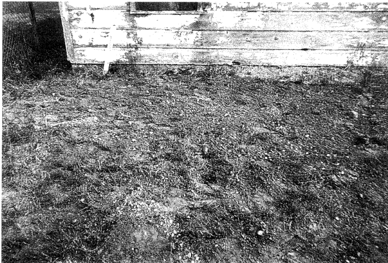
Photograph No.: 4 Contract No.: DACW31-95-D-0097 Location: Pedricktown U.S. Army Reserve Center Photographer: D. Mothershead Description: Site after backfilling UST excavation at Building No. 229. Direction: East.
