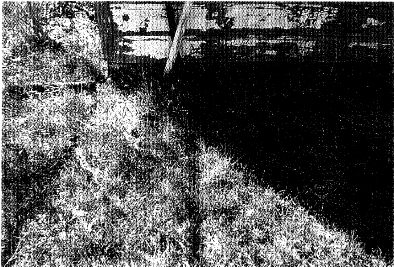
Photograph No.: 1 Contract No.: DACW31-95-D-0097 Earth Tech Job No. 21574 Location: Pedricktown U.S. Army Reserve Center D.O. No.: 015 Photographer: D. Mothershead Date: 5/12/96 Description: Site prior to excavation of UST at Building No. 229. Direction: East.
