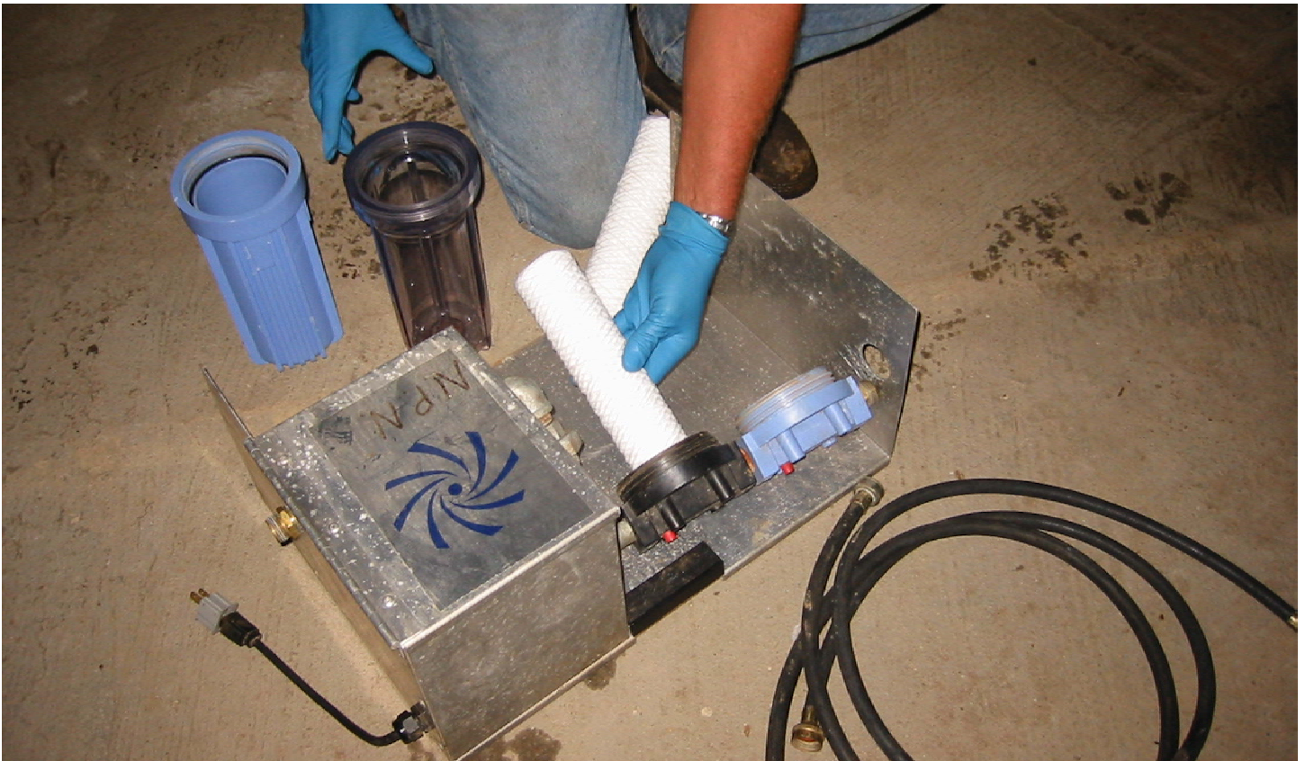
Photograph 33. Building 105 SAFR. Typical 50 micron filter assembly, September 2002.
