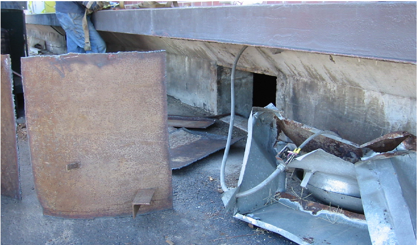
Photograph 27. Building 105 SAFR. Typical metal from Bullet Pit backstop awaiting load-out to recycler, September 2002.
