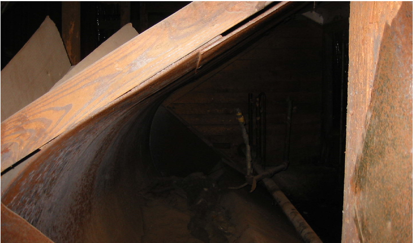
Photograph 15. Building 105 SAFR. End on view of Bullet Pit metal backstop showing curvature, September 2002.
