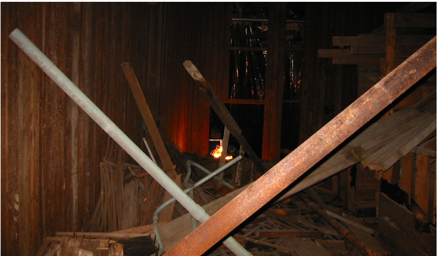
Photograph 16. Building 105 SAFR. Debris (metal pipe, wood, plastics) behind range, September 2002.
