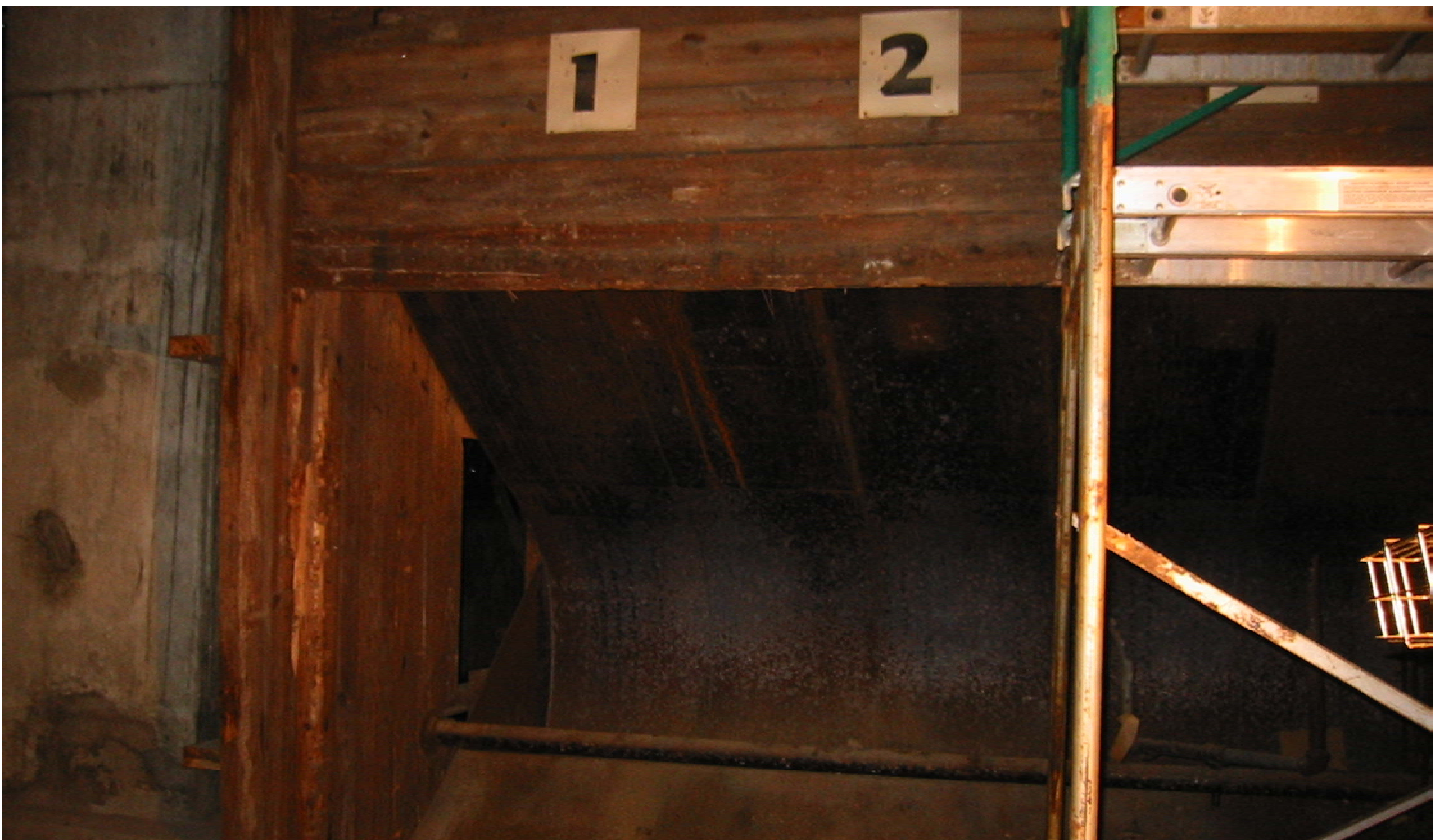
Photograph 14. Building 105 SAFR. Typical scarification evidence on Bullet Pit backstop and of wood framing, September 2002.
