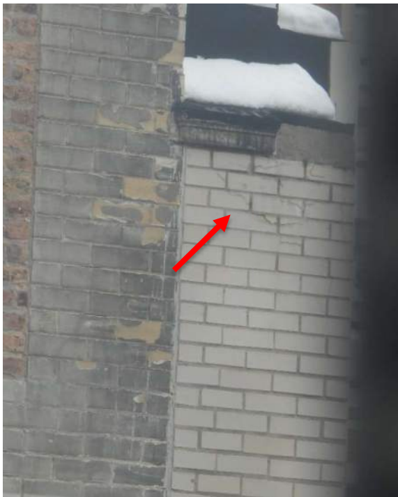
Photo 15. Deteriorated brick at southeast corner of Floor 15. This area was subsequently meshed.
