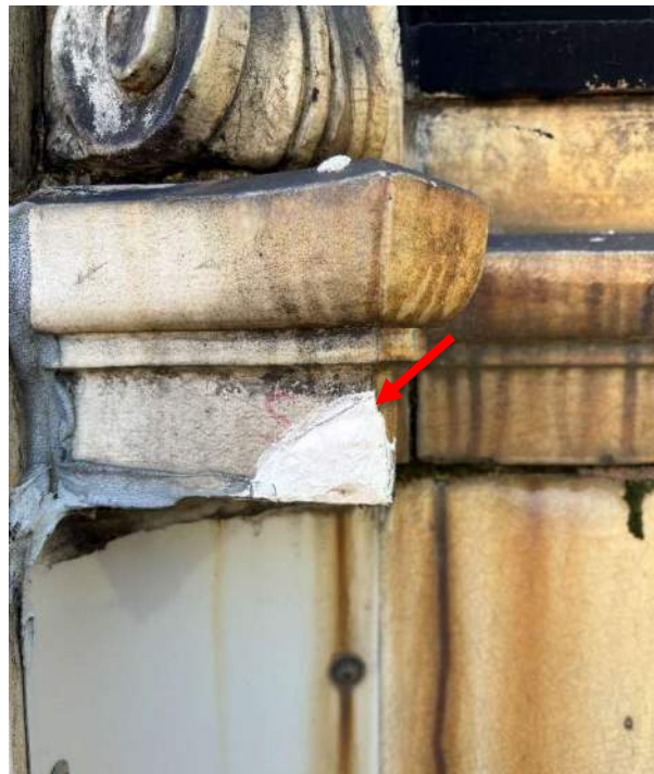
Photo 12. Sealed spall at terra cotta unit
