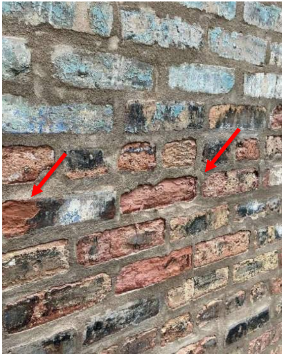
Photo 17. Deteriorated brick at west elevation
