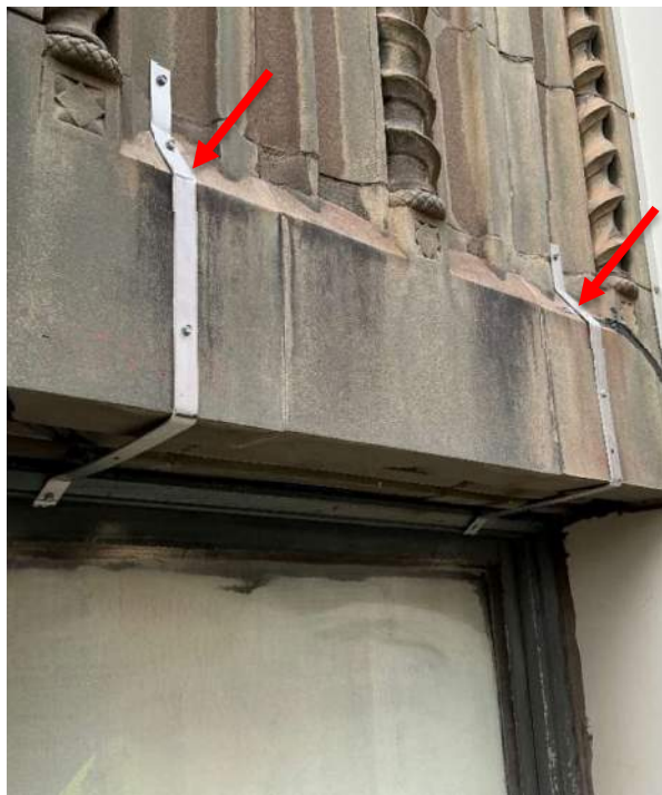
Photo 25. Typical cracked terra cotta metal strap stabilization repair
