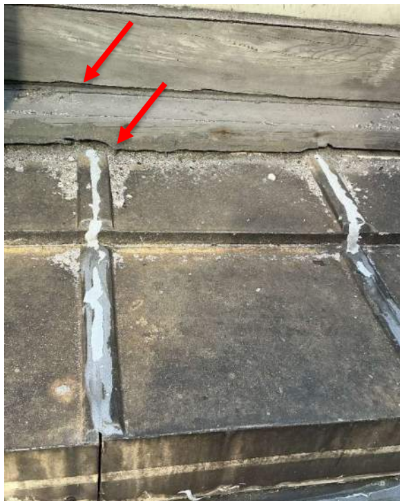
Photo 21. Deterioration of wood sill and sash at window
