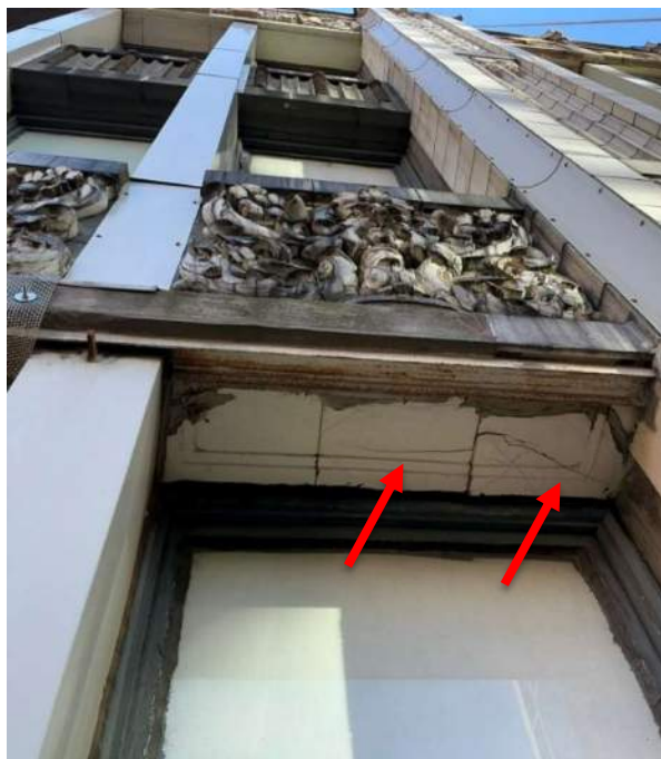
Photo 7. Ornamental spandrel at 14 th floor North Elevation (cracks noted on underside of window head units) – subsequently strapped
