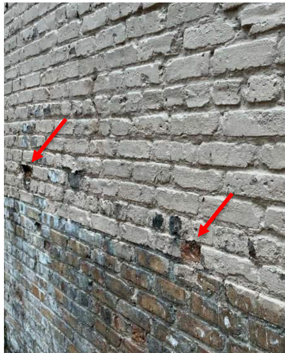
Photo 16. Spalled brick at west elevation
