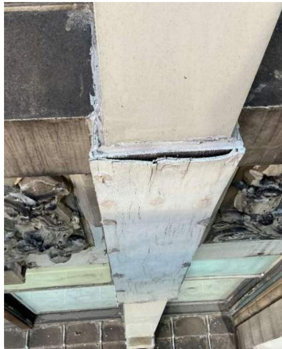
Photo 10 Typical weathered deteriorated plywood coverings at previously removed terra cotta units. This condition was subsequently replaced.
