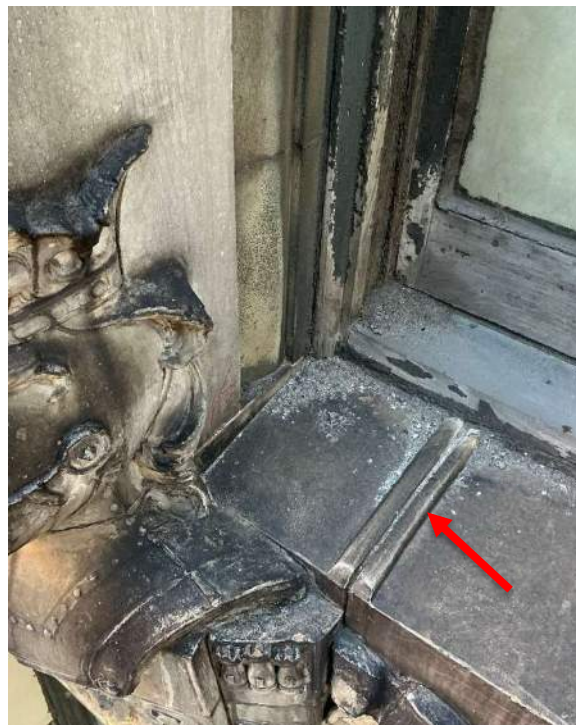
Photo 22. Deteriorated mortar joint at 4 th floor window sill
