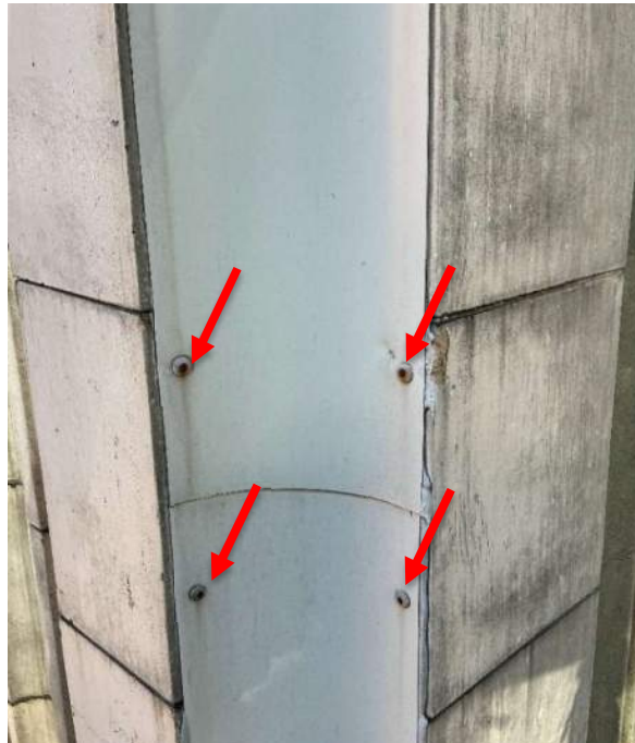
Photo 8. Typical corrodible anchors observed on aluminum sheeting
