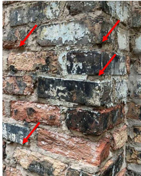
Photo 18. Severely deteriorated mortar joints. Subsequently repointed.
