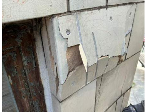
Photo 14. Terra cotta face spall, subsequently rebuilt with white glaze brick.
