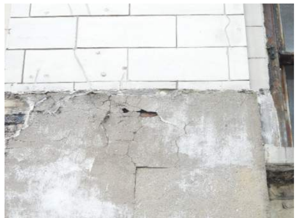
Photo 56. Concrete siding that has spalled and cracked observed from binocular review.
