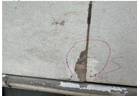
Photo 30. Typical terra cotta glaze spall.
