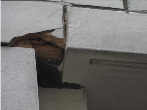
Photo 51. Cracked window header observed from binocular review.
