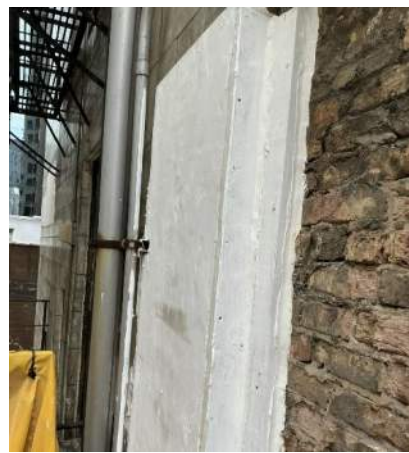
Photo 48. Plywood cover at window jamb cracking at west elevation, 4 th floor.
