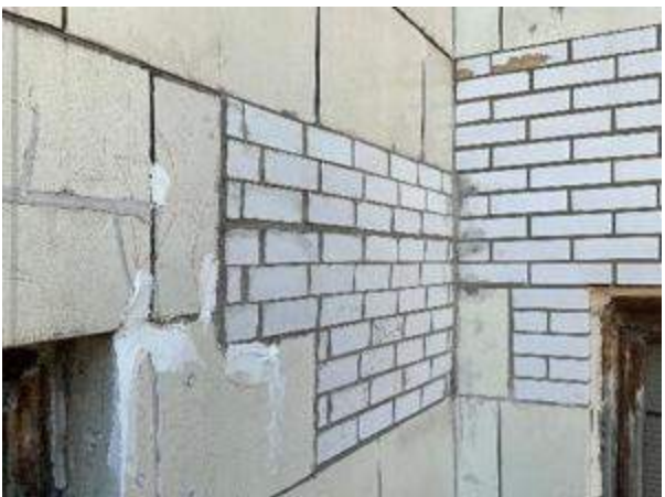
Photo 41. Typical brick infill at locations of terra cotta removal.
