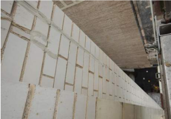
Photo 19. Previously rebuilt brick at the northeast corner of the building.
