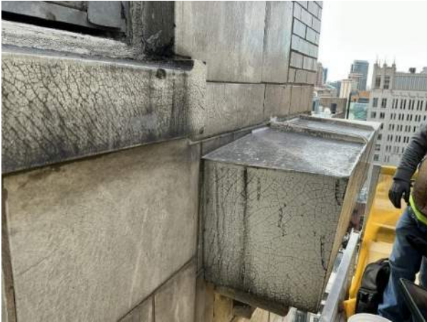
Photo 49. Cracked water table corner pieces at west elevation, 18 th floor removed in 2026 (see next photo for completed repair)
