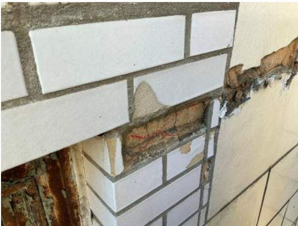
Photo 21. Typical spall at the white glaze brick infill, subsequently replaced in kind.
