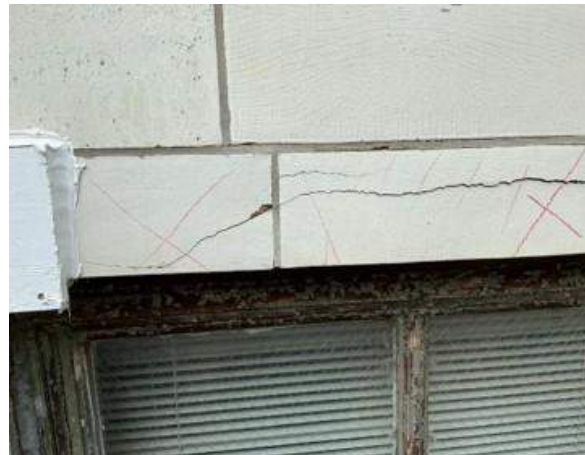
Photo 28. Severe cracking at terra cotta window head units, subsequently removed and covered with plywood.
