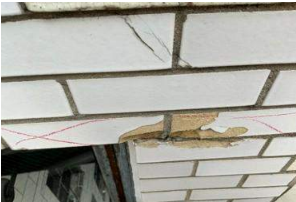
Photo 29. Typical glaze spalling on white glaze masonry infill.
