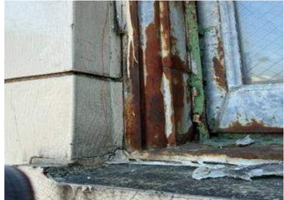
Photo 26. Corrosion at metal window frame.
