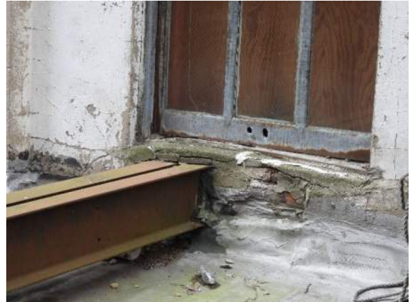
Photo 52. Cracked window sill observed from binocular review.
