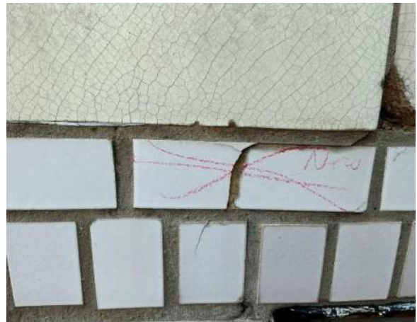
Photo 22. Cracked white glaze brick at masonry infill, subsequently replaced in kind.
