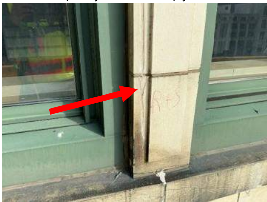
Photo 9. Typical terra cotta mullion on the east elevation, with crack noted by red arrow, subsequently routed and sealed.
