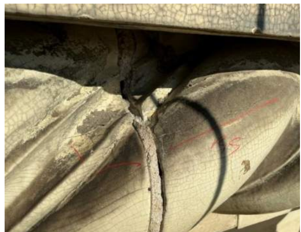
Photo 12. Deteriorated mortar joints at cornice torsade at the south elevation.
