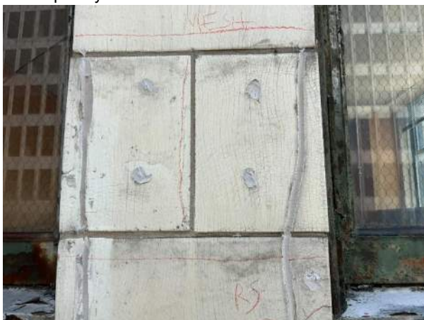
Photo 11. Previous terra cotta repairs at column units in poor condition.
