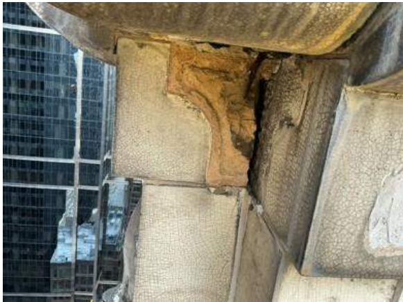
Photo 7. 22 nd floor water table with missing terra cotta portion with corroded steel tie shown, exposed terra cotta subsequently covered with plywood.
