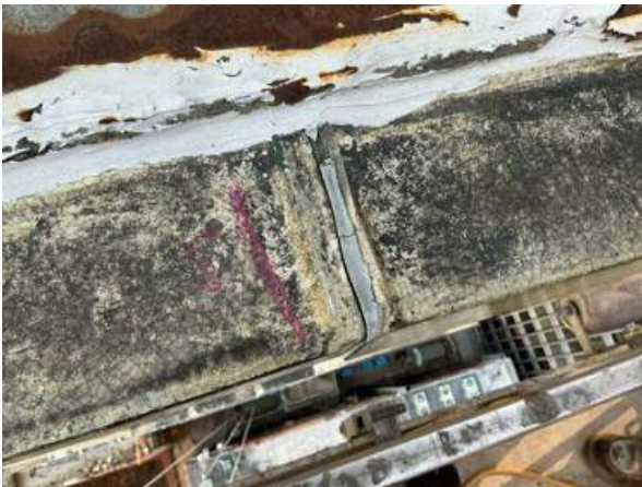
Photo 27. Typical debonded skyward sealant joint at terra cotta window sill, subsequently replaced in kind.
