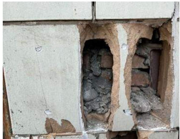
Photo 18. Exposed terra cotta core due to face spall, subsequently rebuilt with white glaze brick.
