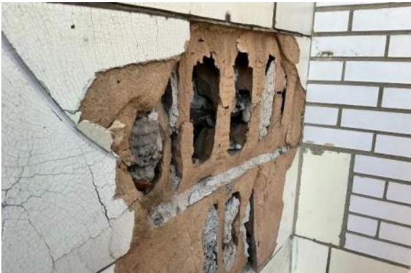
Photo 15. Exposed terra cotta core due to face spall, subsequently rebuilt with white glaze brick.
