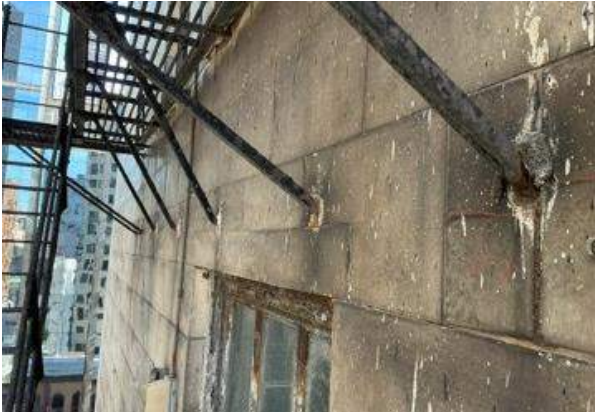
Photo 25. Spalling terra cotta at west elevation fire escape anchorage.
