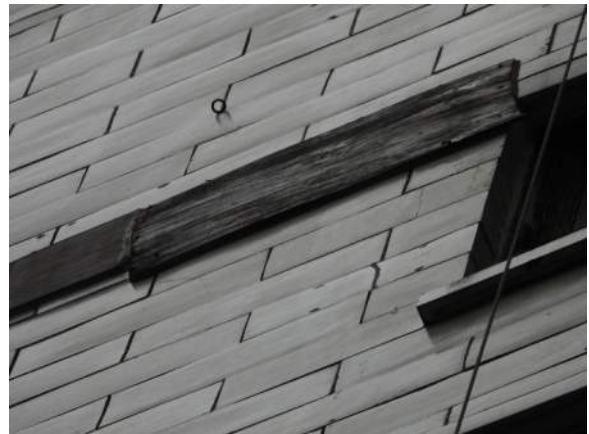
Photo 54. Existing plywood that needs be repainted observed from binocular review.
