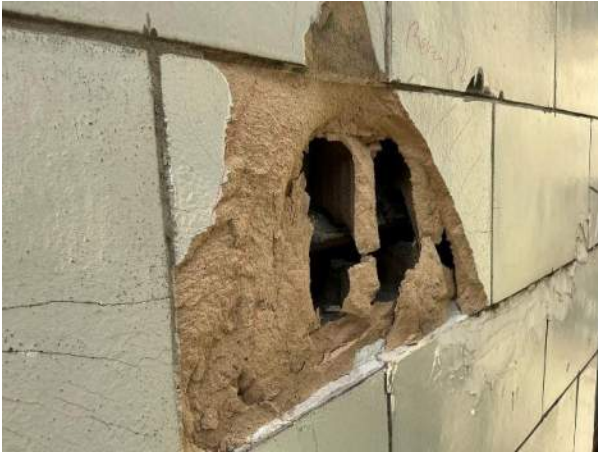
Photo 13. Exposed terra cotta core due to face spall, subsequently rebuilt with white glaze brick.
