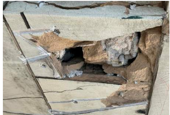
Photo 16. Exposed terra cotta core due to face spall, subsequently rebuilt with white glaze brick.
