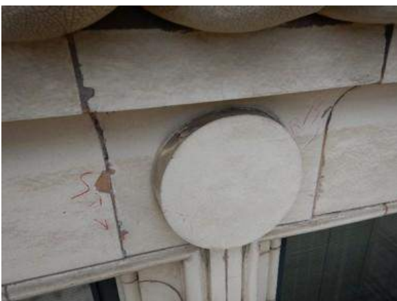
Photo 5. Terra cotta capping at columns below 21 st floor water table (2021 photo for reference only, repairs have been completed).
