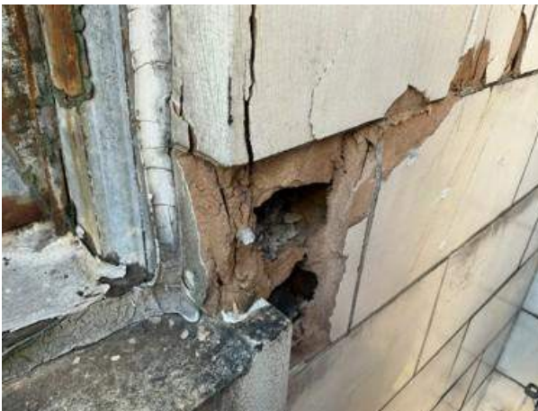
Photo 17. Exposed terra cotta core due to face spall, subsequently rebuilt with white glaze brick.
