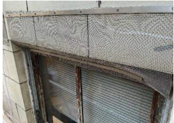
Photo 40. Typical mesh covering at removed terra cotta header unit.
