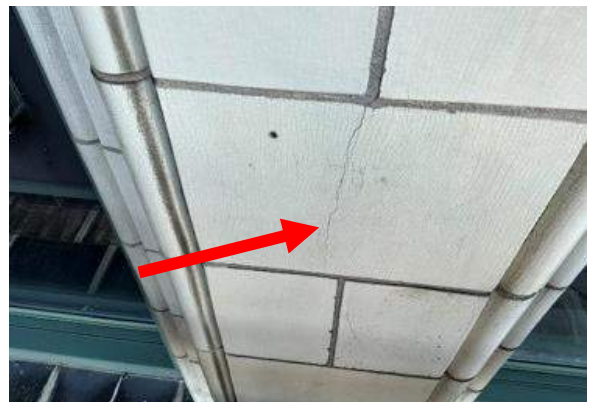
Photo 10. Typical cracked terra cotta mullion units on the south elevation, subsequently routed and sealed.
