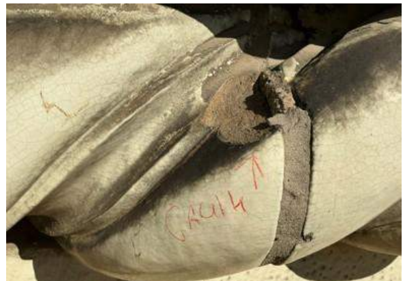
Photo 4. Spall along torsade on the 21 st floor water table.
