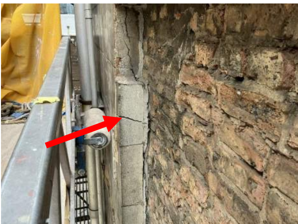
Photo 47. Window jamb cracking at west elevation, 4 th floor.
