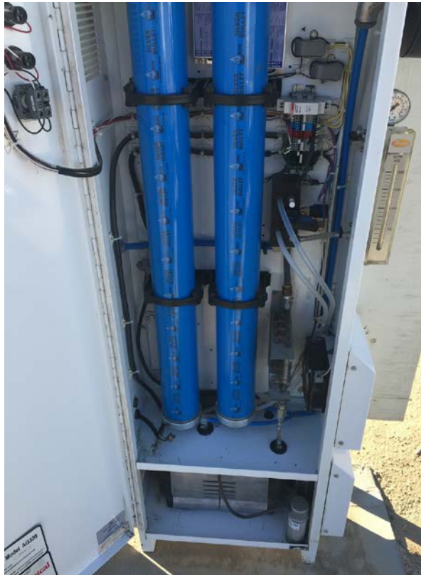
Figure 2. Inside of cabinet AOP technology
