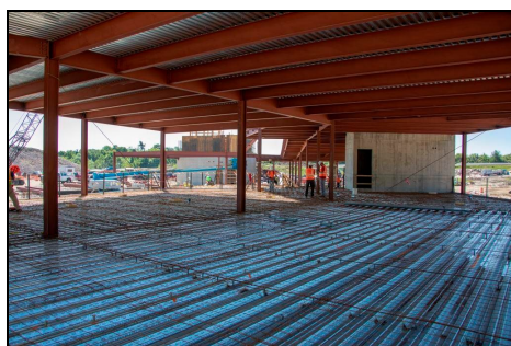
A view of the commercial building mezzanine level deck prior to the concrete pour of the floor. (Courtesy of Revette Studio)
