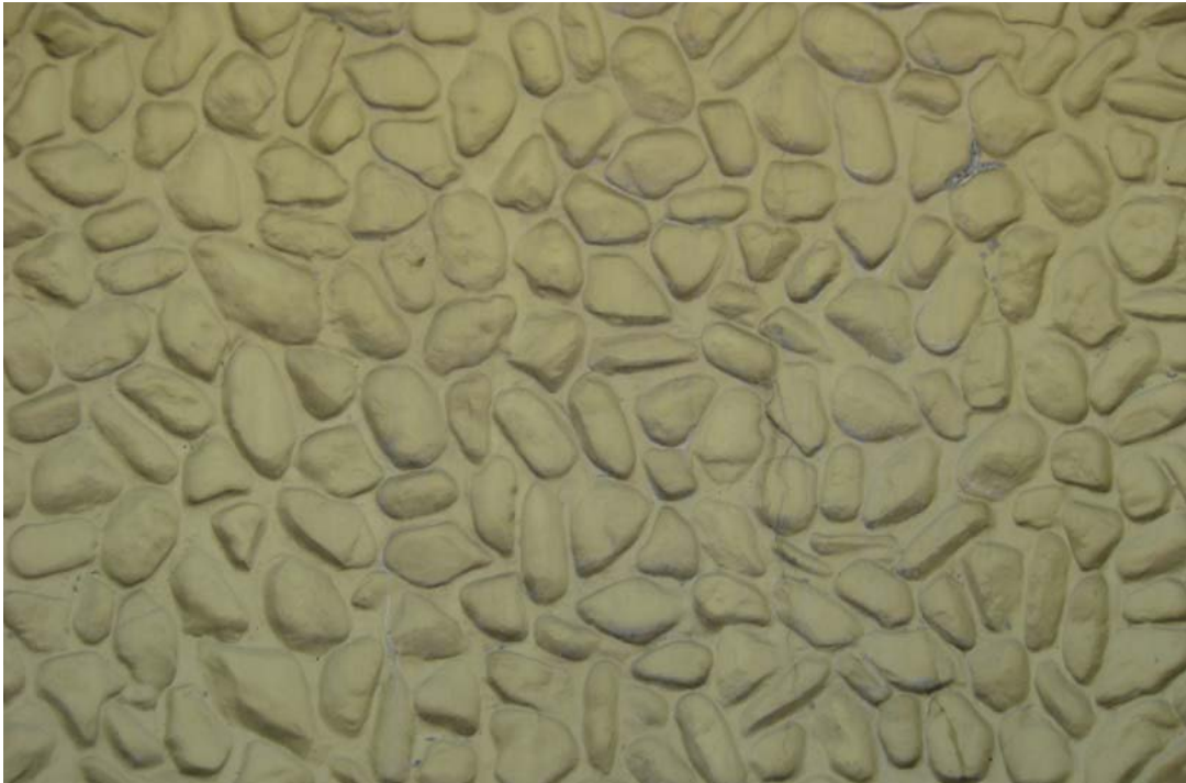
Image 22: Close-up view of the typical exterior wall finish. The pre-cast concrete panels have a pebble texture.
