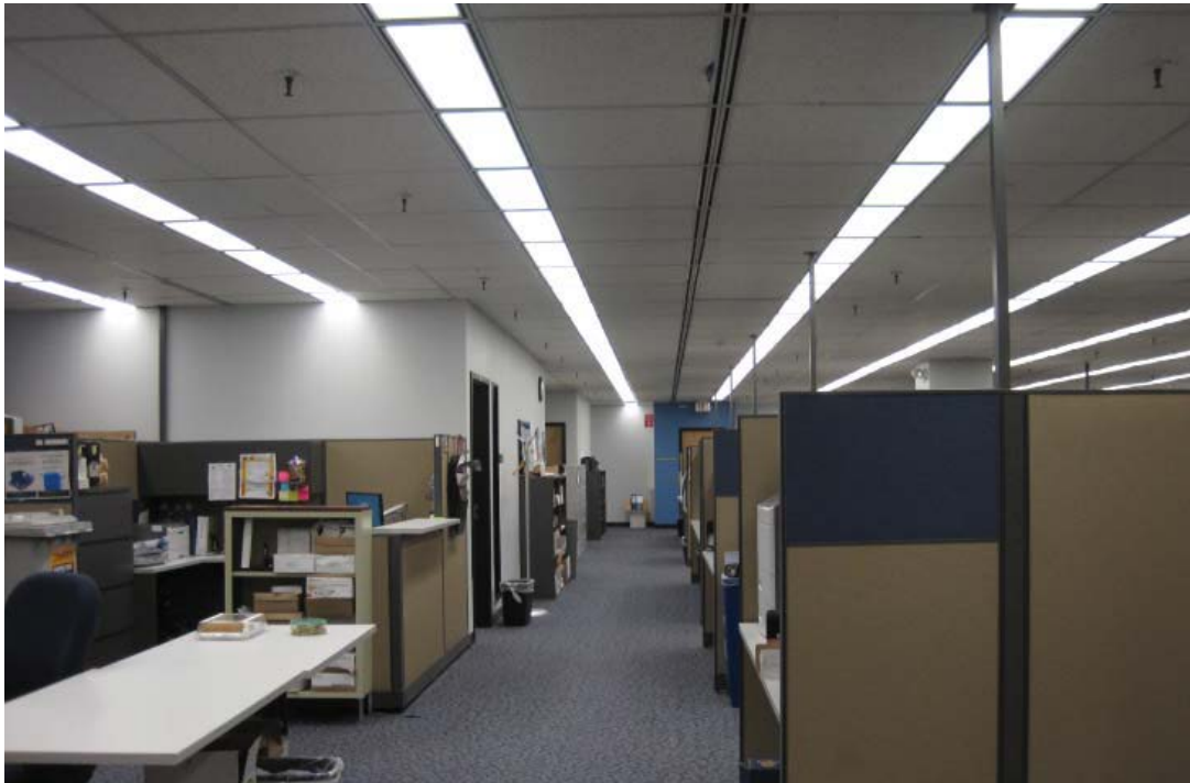
Image 36: A typical office area on the third floor. The suspended ceiling appears to be original, but other interior finishes have been replaced.
