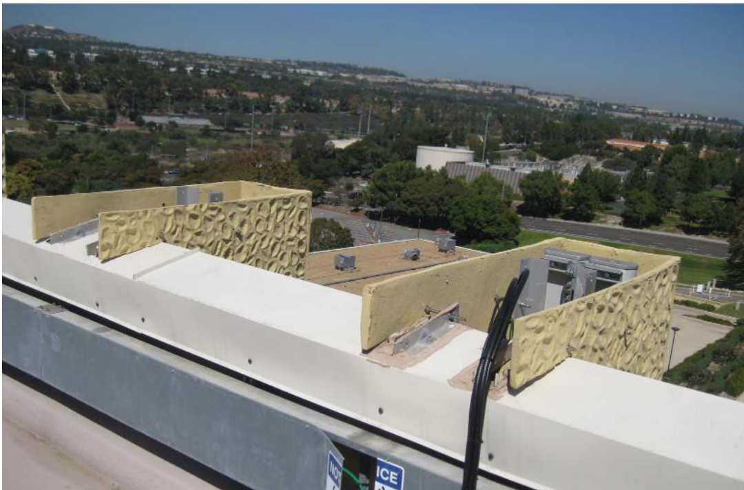
Image 43: A detail of the added fiberglass equipment screens from above.
