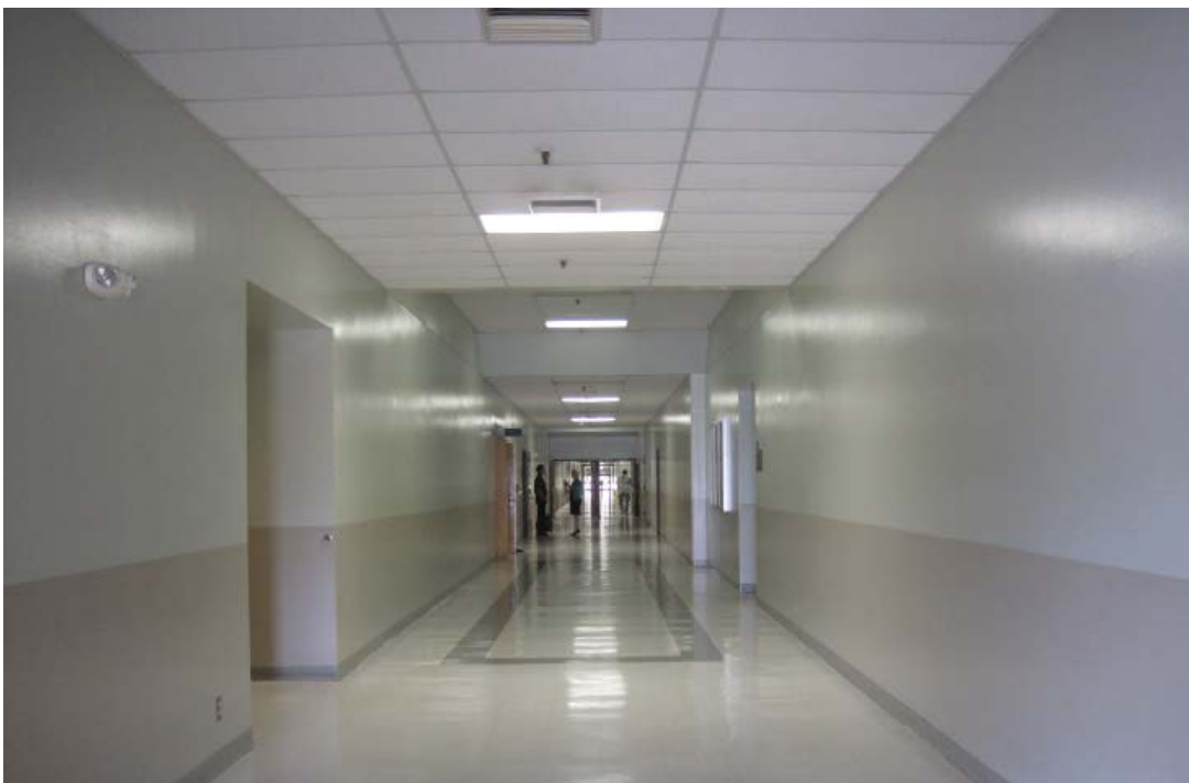
Image 31: A typical corridor on the second floor. The interior finishes in this corridor have been replaced.
