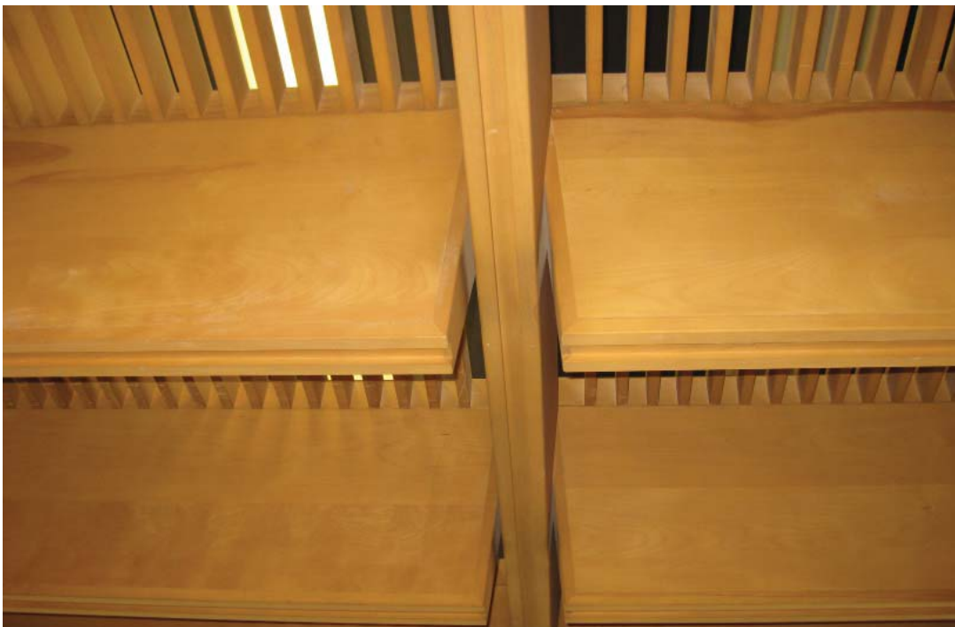
Image 41: A detail of the original wood ceiling finish at the fourth floor lobby.
