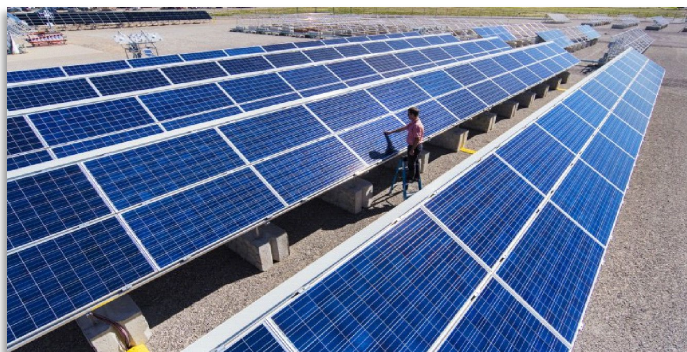
PHOTO 1. EXAMPLE GROUND-MOUNTED SOLAR ARRAY
