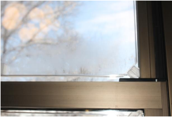
(c) Window attachments in the corners of the window lite hold the panel in place.
