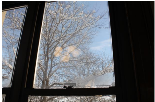
(b) Condensation on the first-floor windows.
