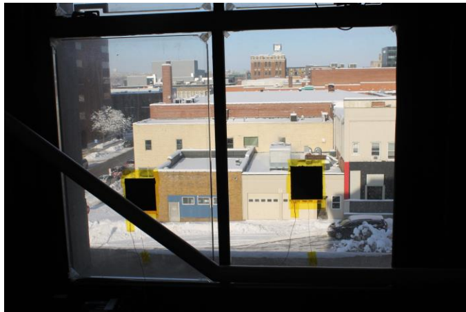
Figure 5. Window with heat flux sensors installed. The operable window sash had four glass lites. The insulation panel technology was installed on three of the four glass lites; both upper lites are outside the image frame, and the left lite is shown in this image. The insulation panel technology was not installed on the right lite so that a heat flux sensor could simultaneously measure the baseline IGU and the IGU that has the insulation panel technology installed.
