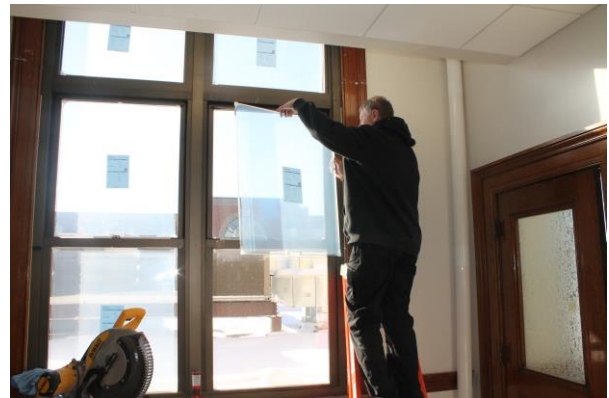
(b) Window lites were premeasured, and the insulation panel was fabricated to size.
