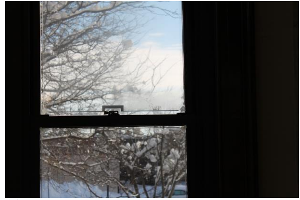
(b) Window panels are presented around the window lock in a first-floor office.
