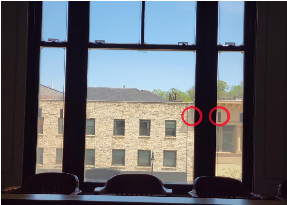
Figure 17. Transparent spacers at the Eau Claire Courthouse. The left red circle is the clear spacer. The right red circle is the milky-white original spacers.
