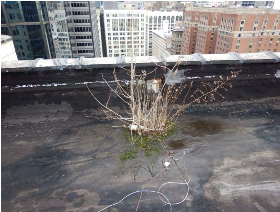
Clogged upper roof drain with vegetation
