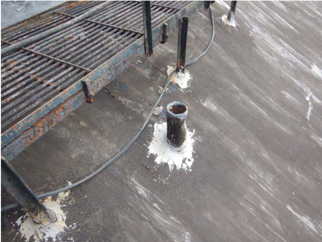
Failed roofing membrane around stair supports and vent stack
