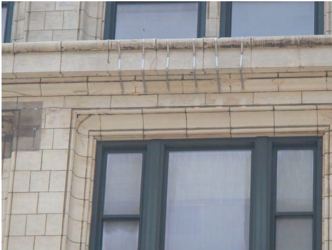
Overview of steel straps installed at water table and cracking at terra cotta lintel units
