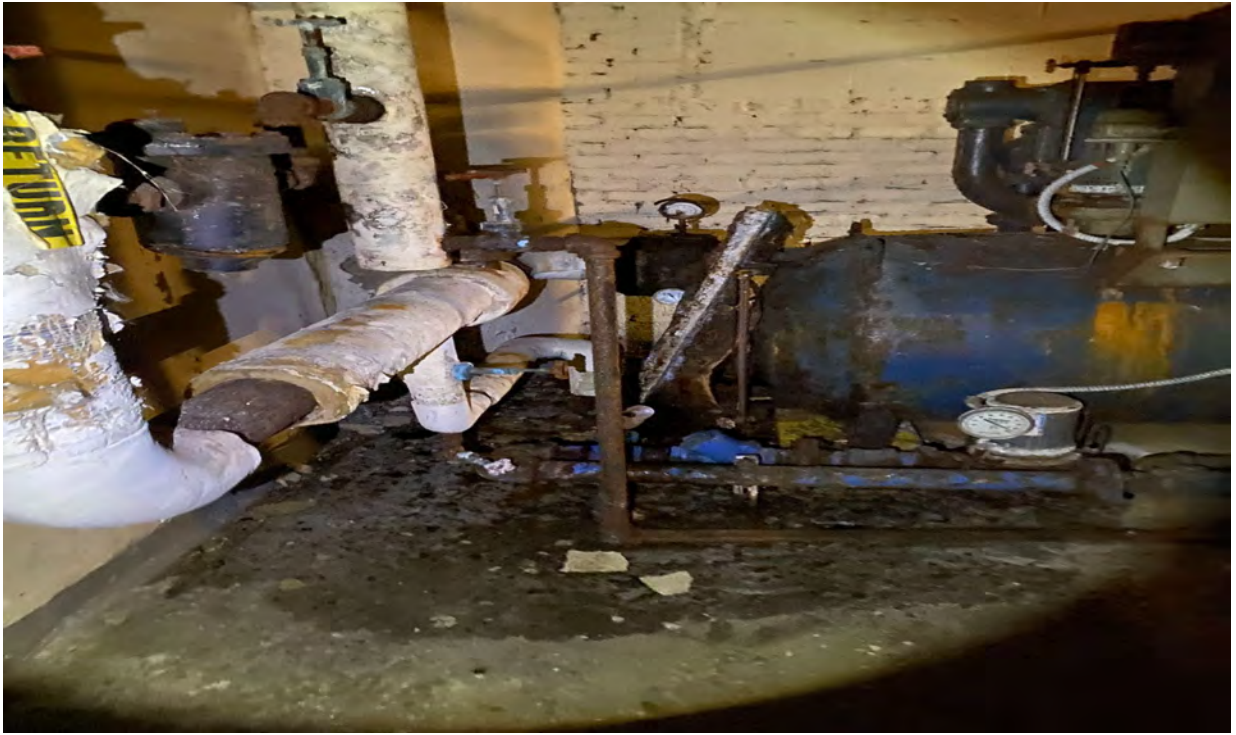
Basement 3 - Existing Condensate tank and pump
