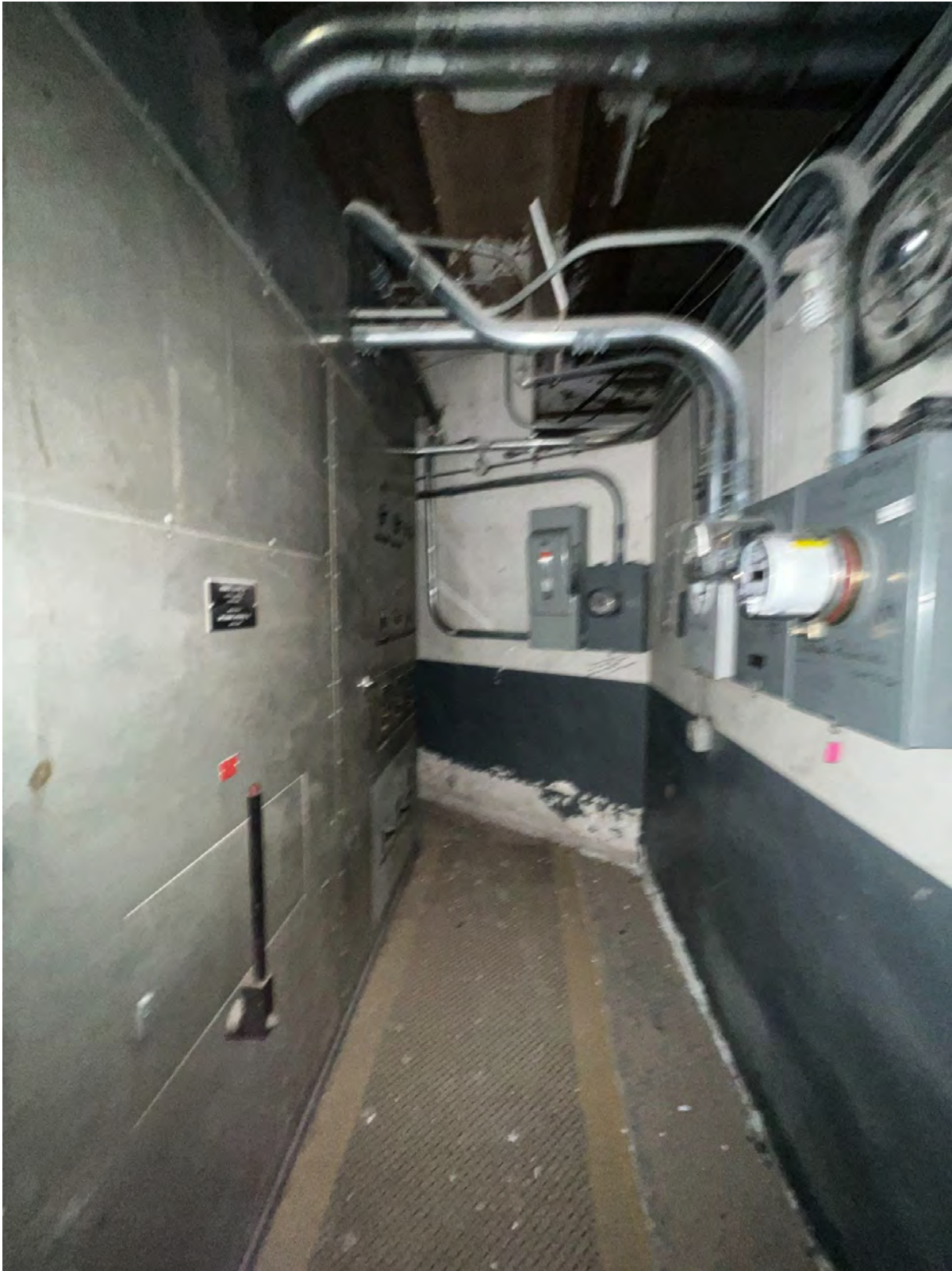
Sub-basement: Existing 120/208v switchboard
