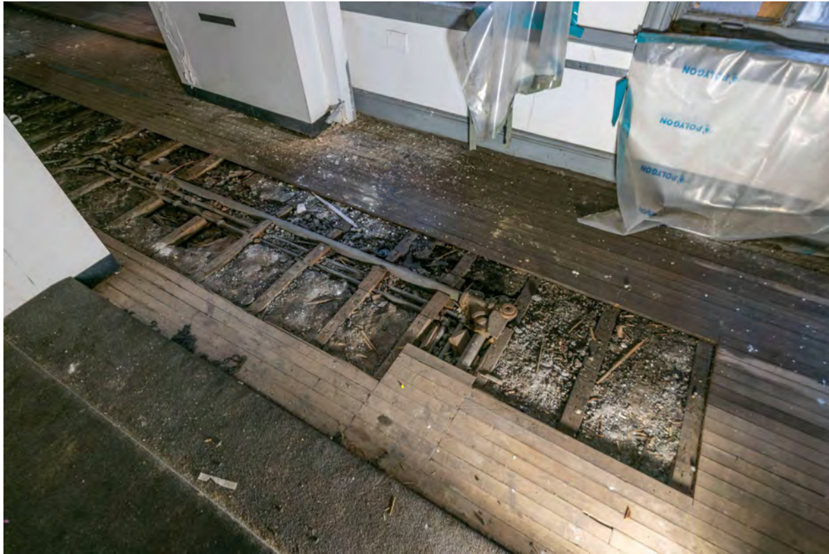
Level 2 Pipe Distribution Between the Flooring and the Top of the Clay Tile Arch
