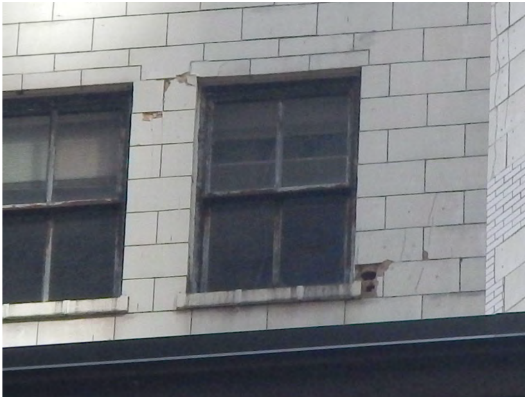
Overview of north elevation with terra cotta spalled units and cracked units
