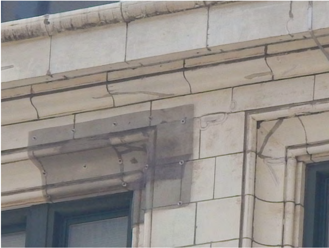
Overview of steel mesh repair effort and crack repair efforts and window lintel
