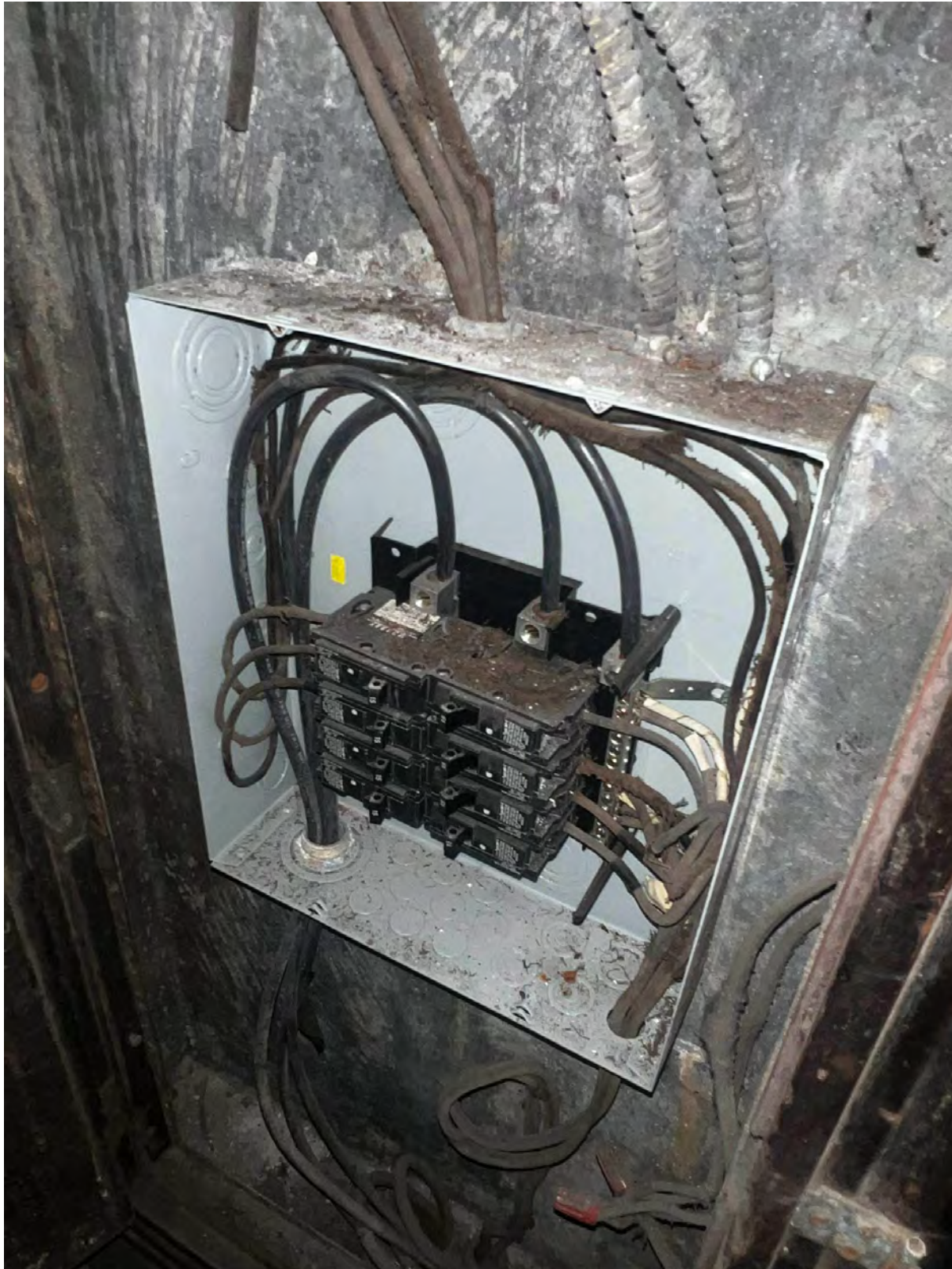
1st Floor: Panelboard with possible cloth wiring.
