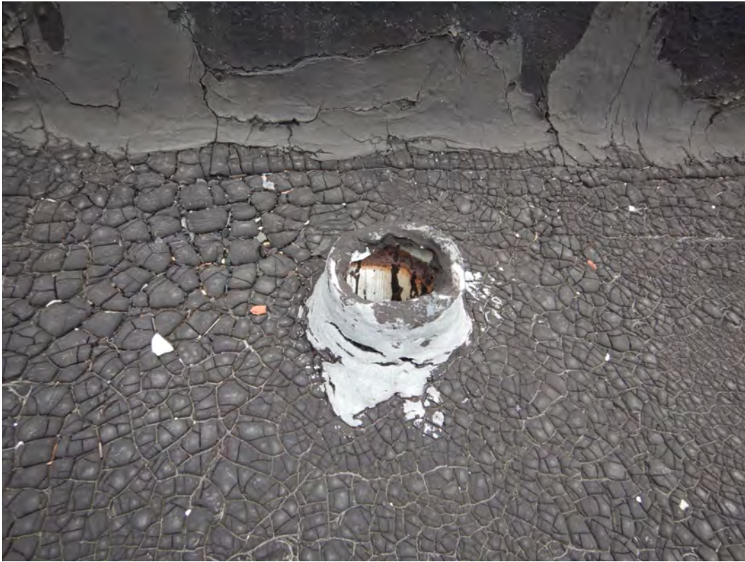
Failed vent stack roofing detail and deteriorated roofing membrane
