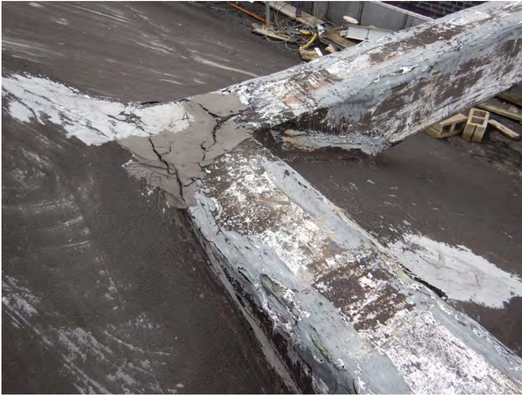
Severely deteriorated horizontal braces intersecting sloped roof
