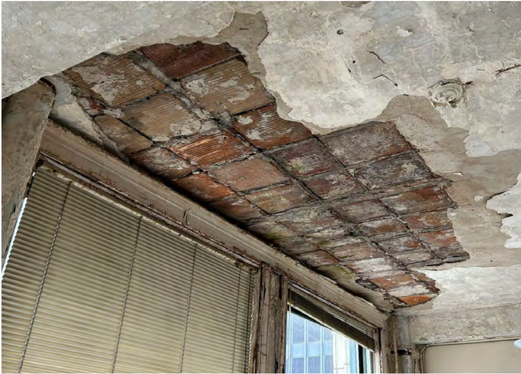
Superstructure: Exposed clay tile arch floor structure at localized area of past water infiltration
