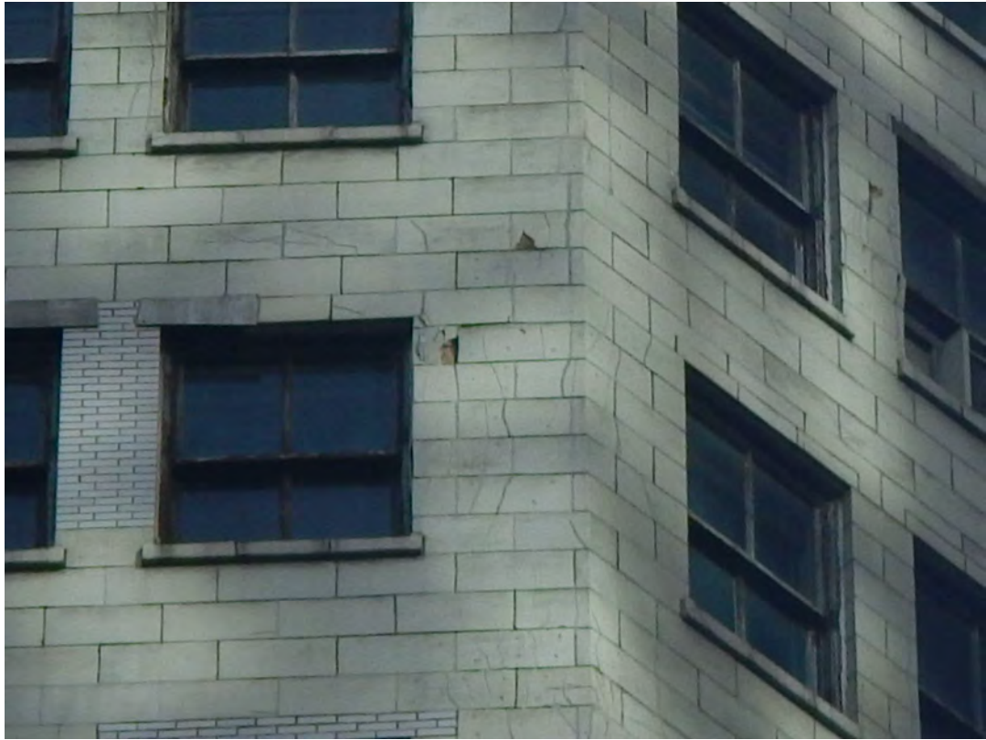
Overview of north elevation with terra cotta spalled units and cracked units
