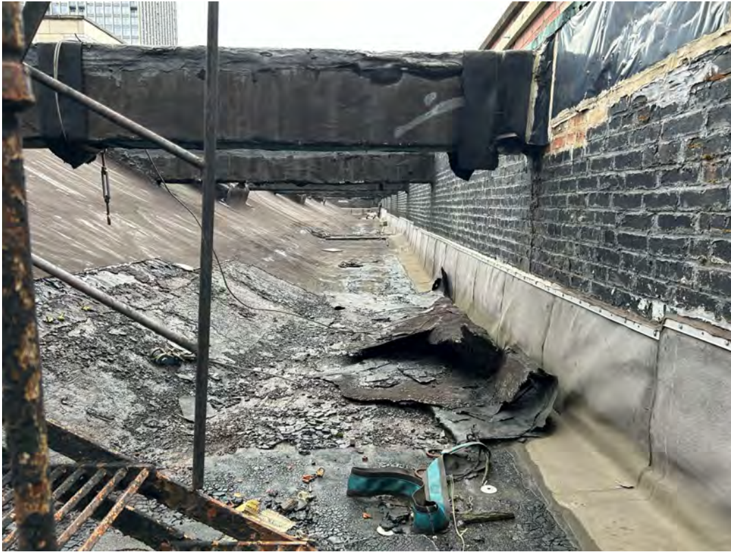
Severely deteriorated roofing membrane at south east corner
