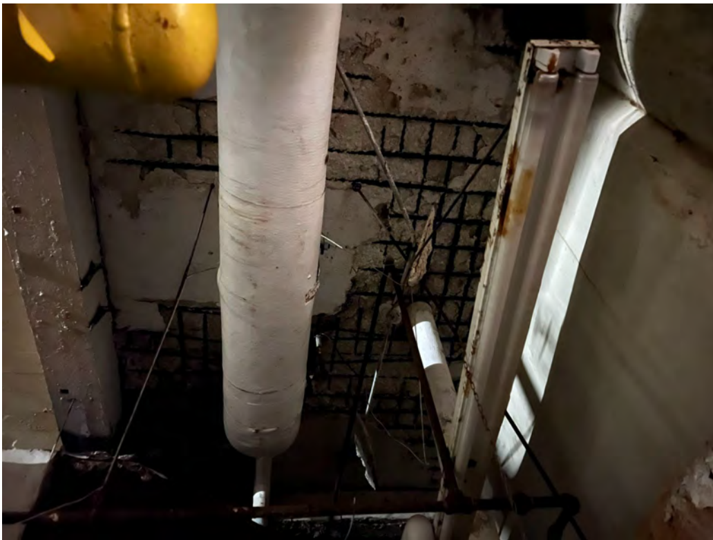
Middle basement slab from below: Area with exposed and corroded rebar
