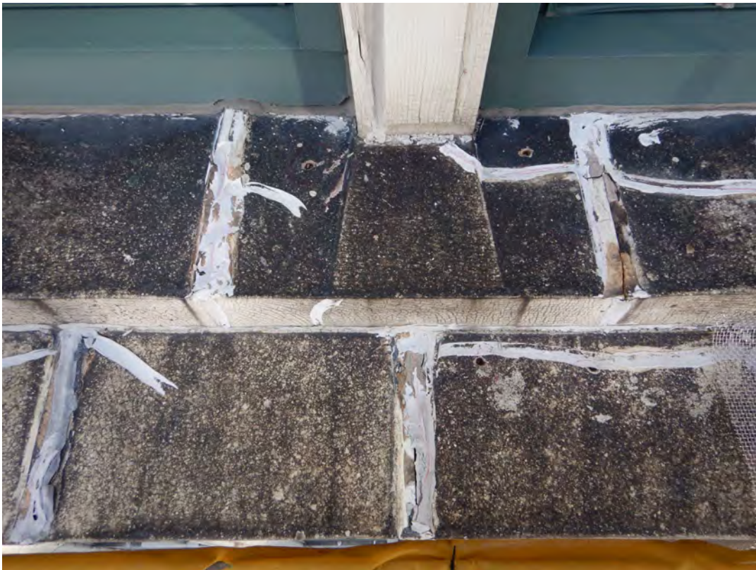
Overview of previous repair efforts and open joint at water table
