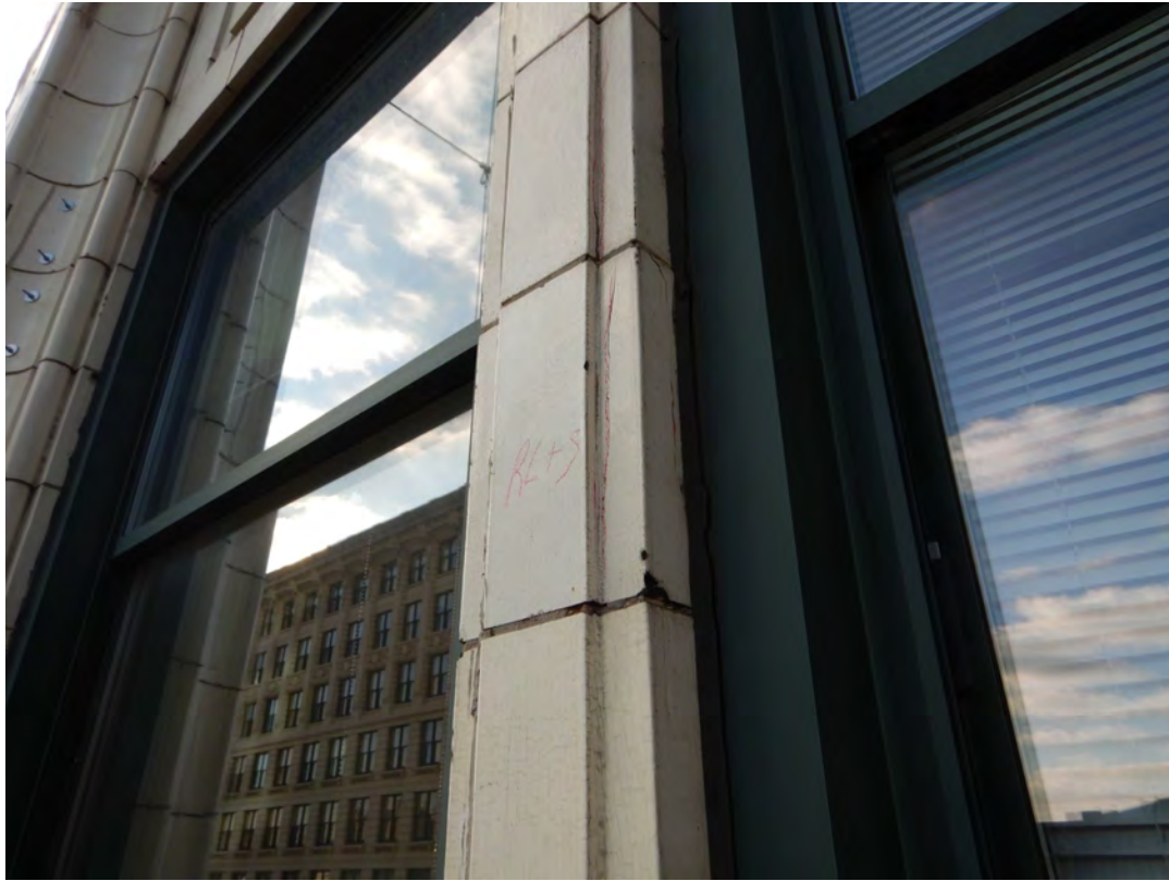
Overview of terra cotta mullion units with newer crack
