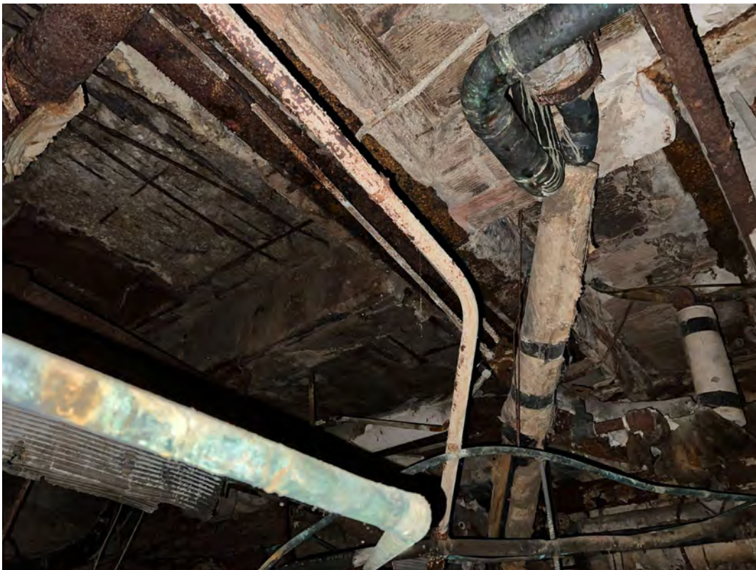
Ground level slab from below: Northwest room, heavy spalling and corroded and displaced rebar
