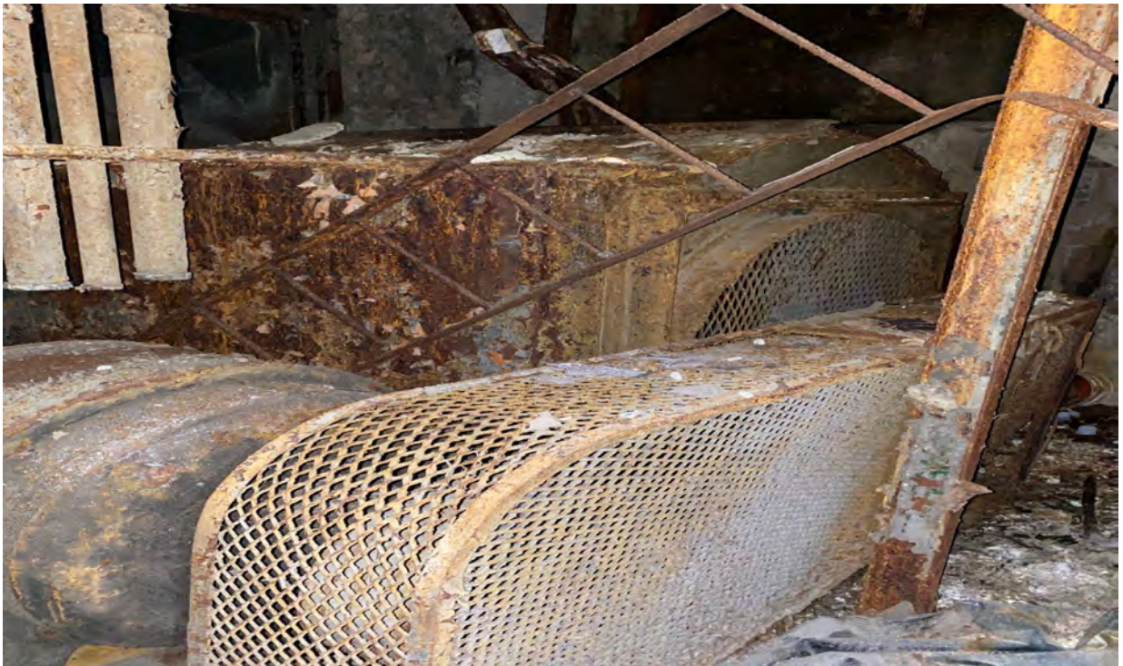
Basement 2 - Existing Outdoor air intake fan
