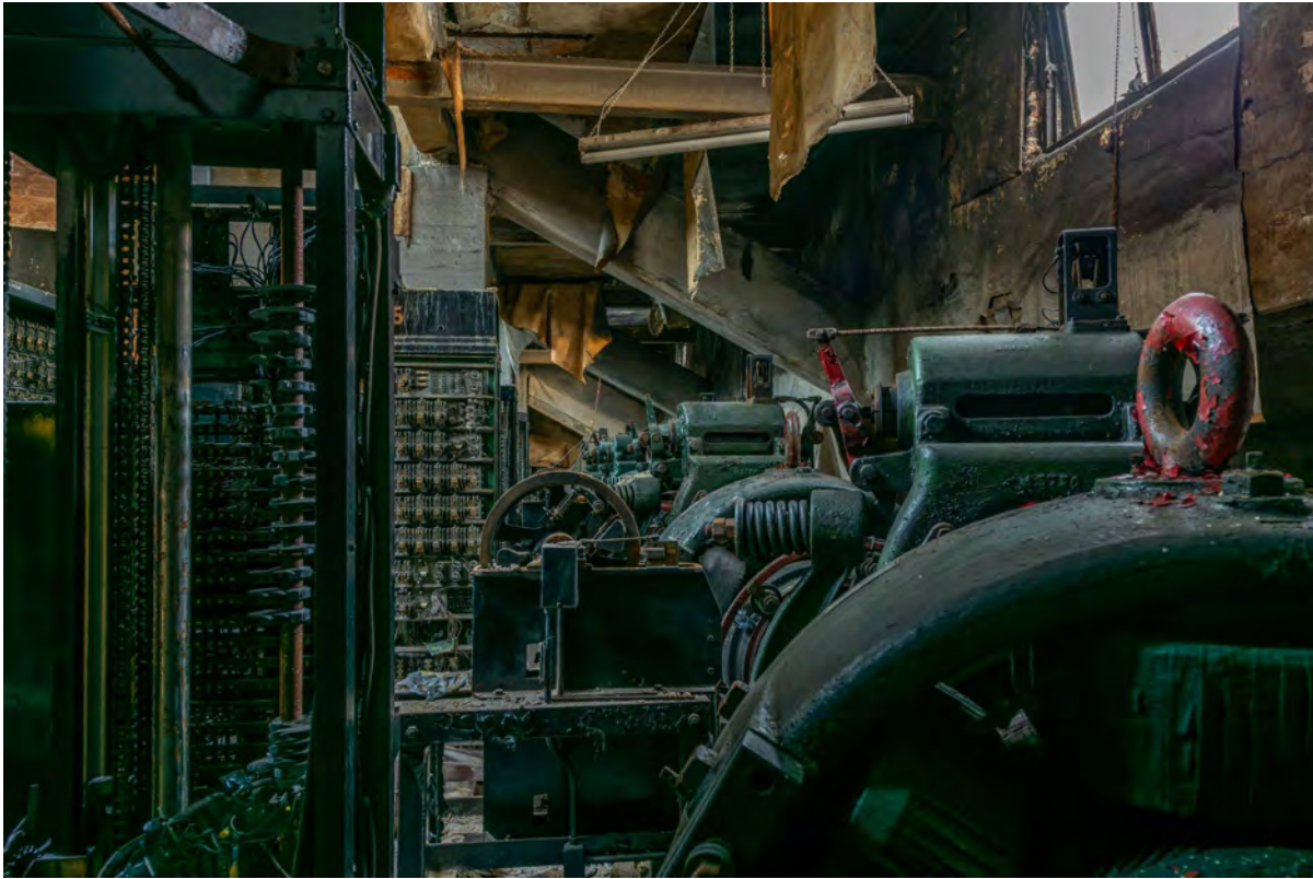
Level 22 Elevator Machine Room
