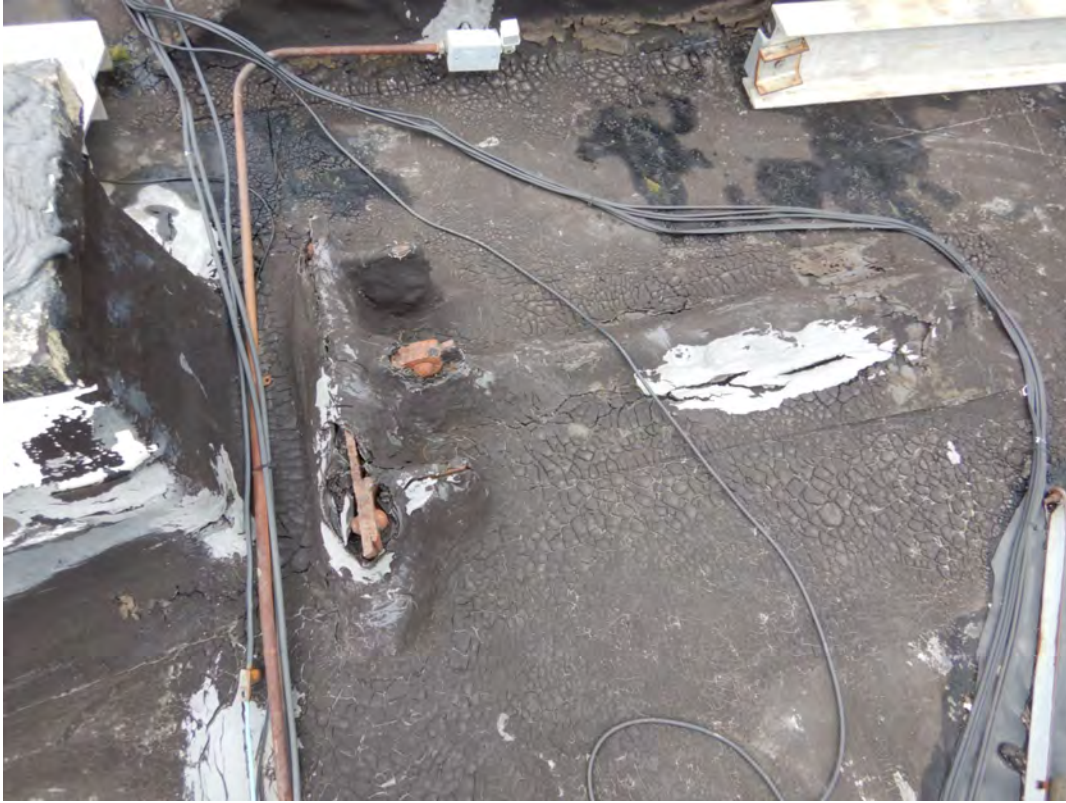
Open tears within the roofing membrane on the upper roof
