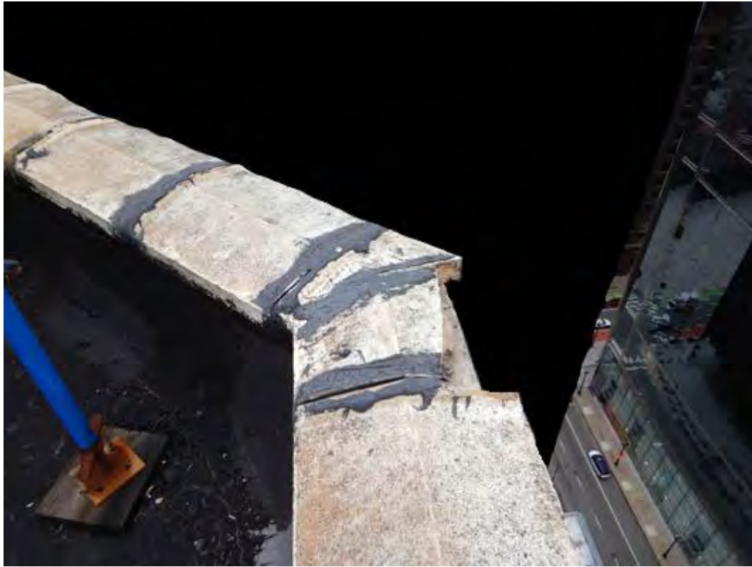
Damaged terra cotta coping
