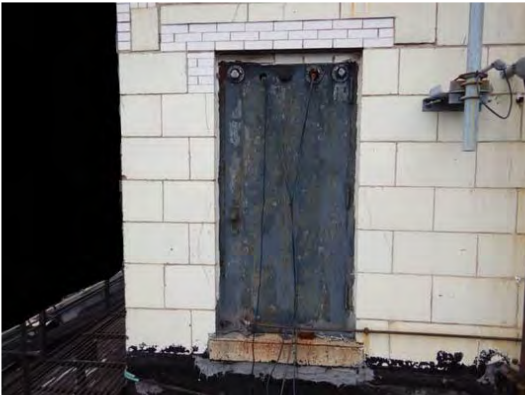
Deteriorated penthouse door and cladding
