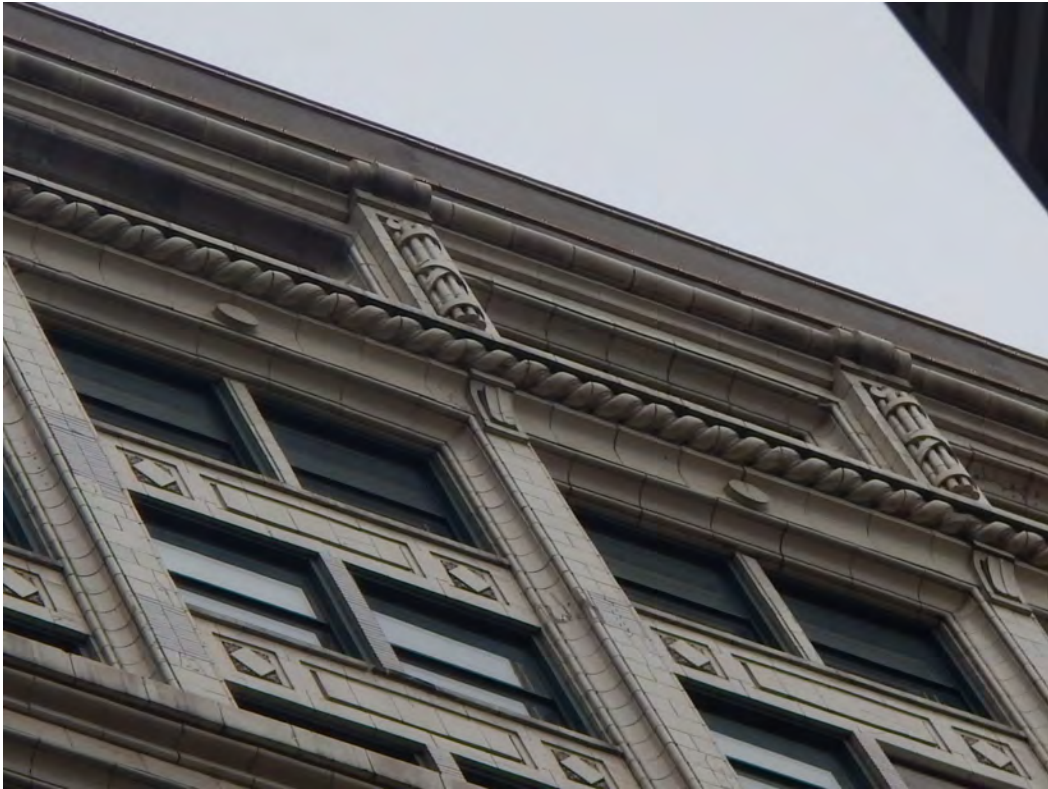
Overview of water tables at upper floors
