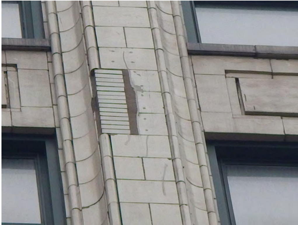
Terra cotta column with various previous repair efforts
