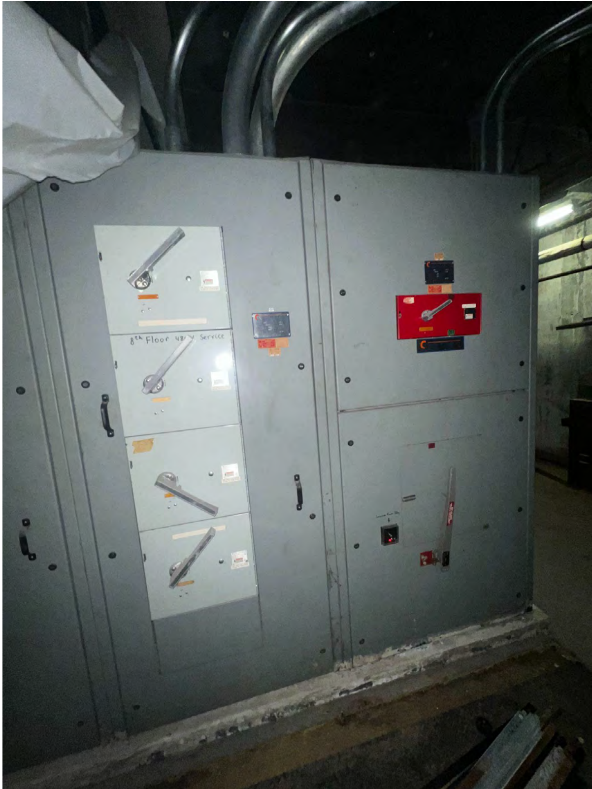
Sub Basement: Existing 480v switchboard
