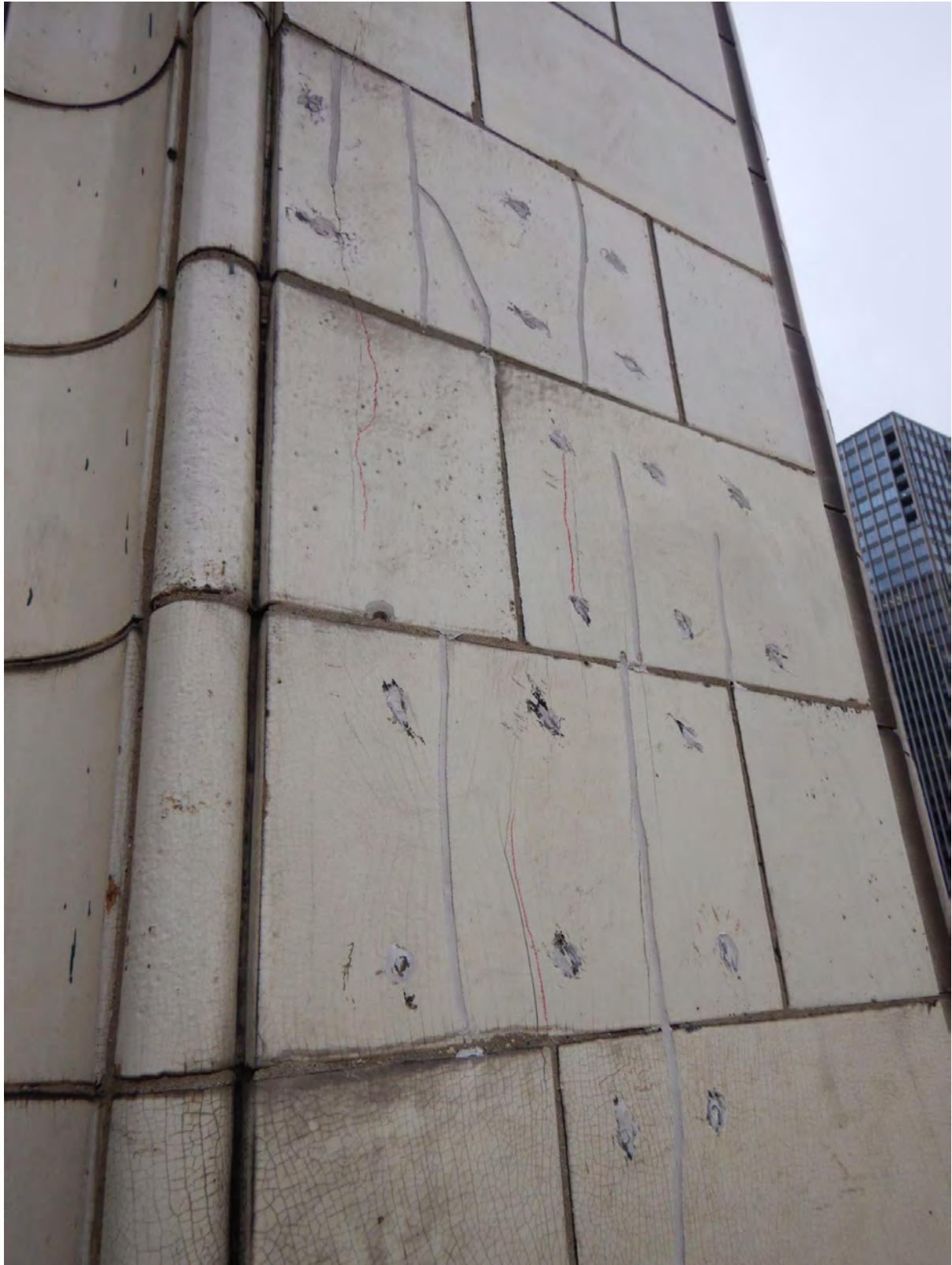
Terra cotta column with various previous repair efforts
