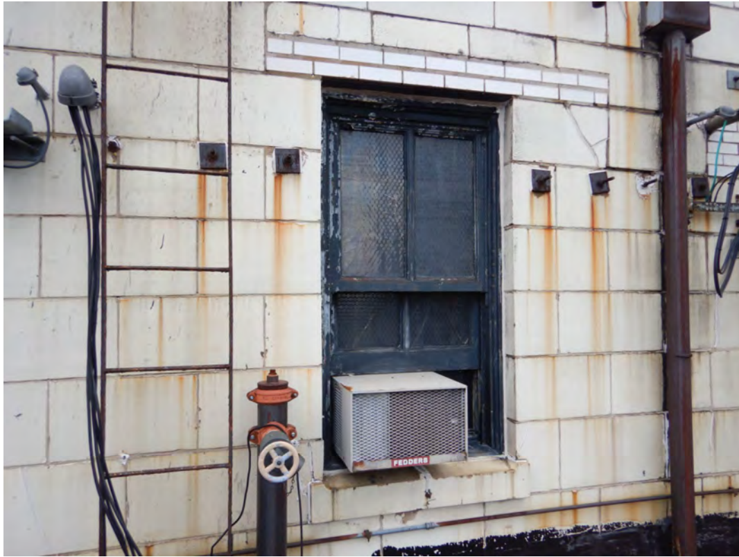
Deteriorated penthouse window and roof ladder
