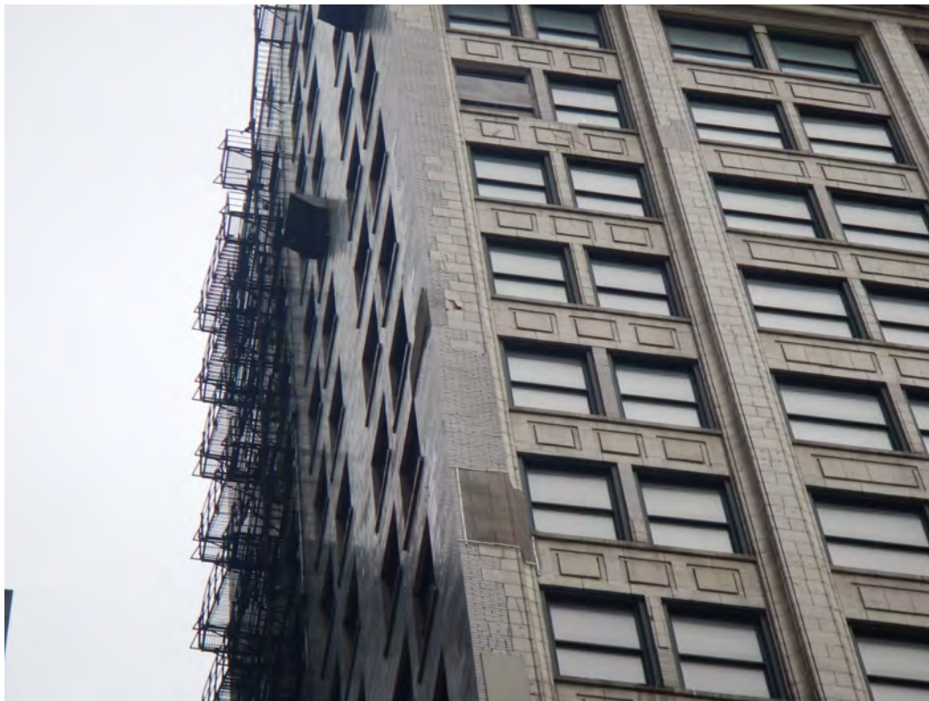
Terra cotta column with various previous repair efforts and new area of spall (dark area at mid-height of west column)
