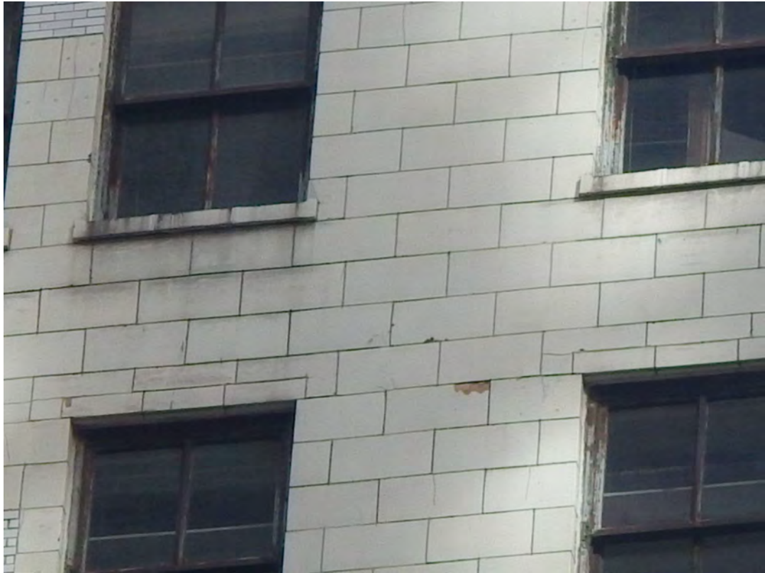
Overview of north elevation with terra cotta spalled units and cracked units
