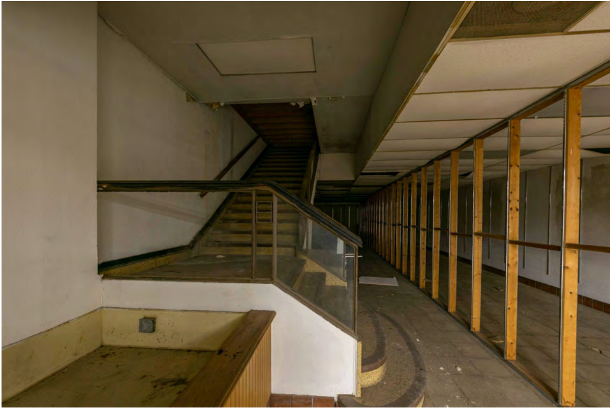
Lower Level 1 Abandoned Stair from 1st Floor
