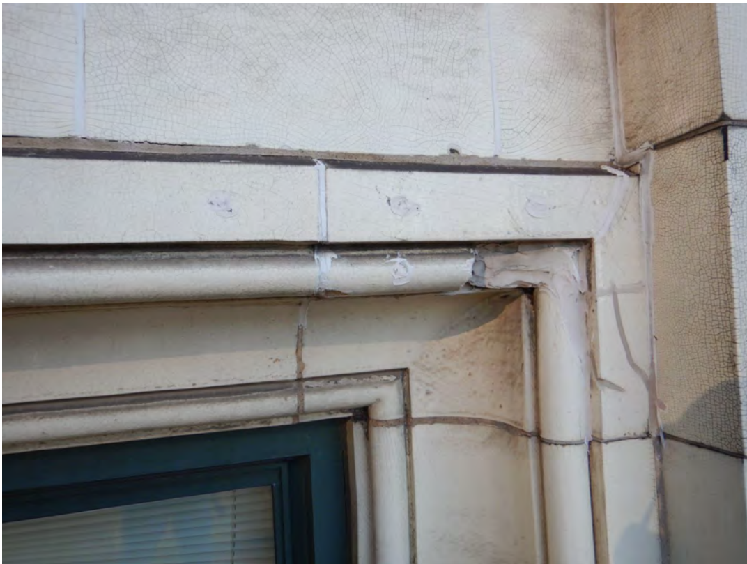
Previous repair efforts at terra cotta window lintel
