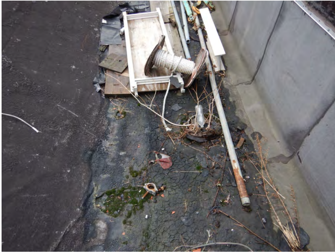
Clogged lower roof drain
