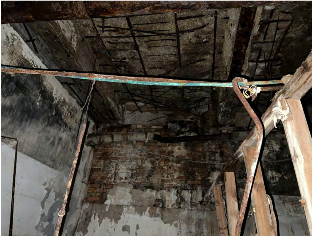
Ground level slab from below: Northwest room, heavy spalling and corroded and displaced rebar
