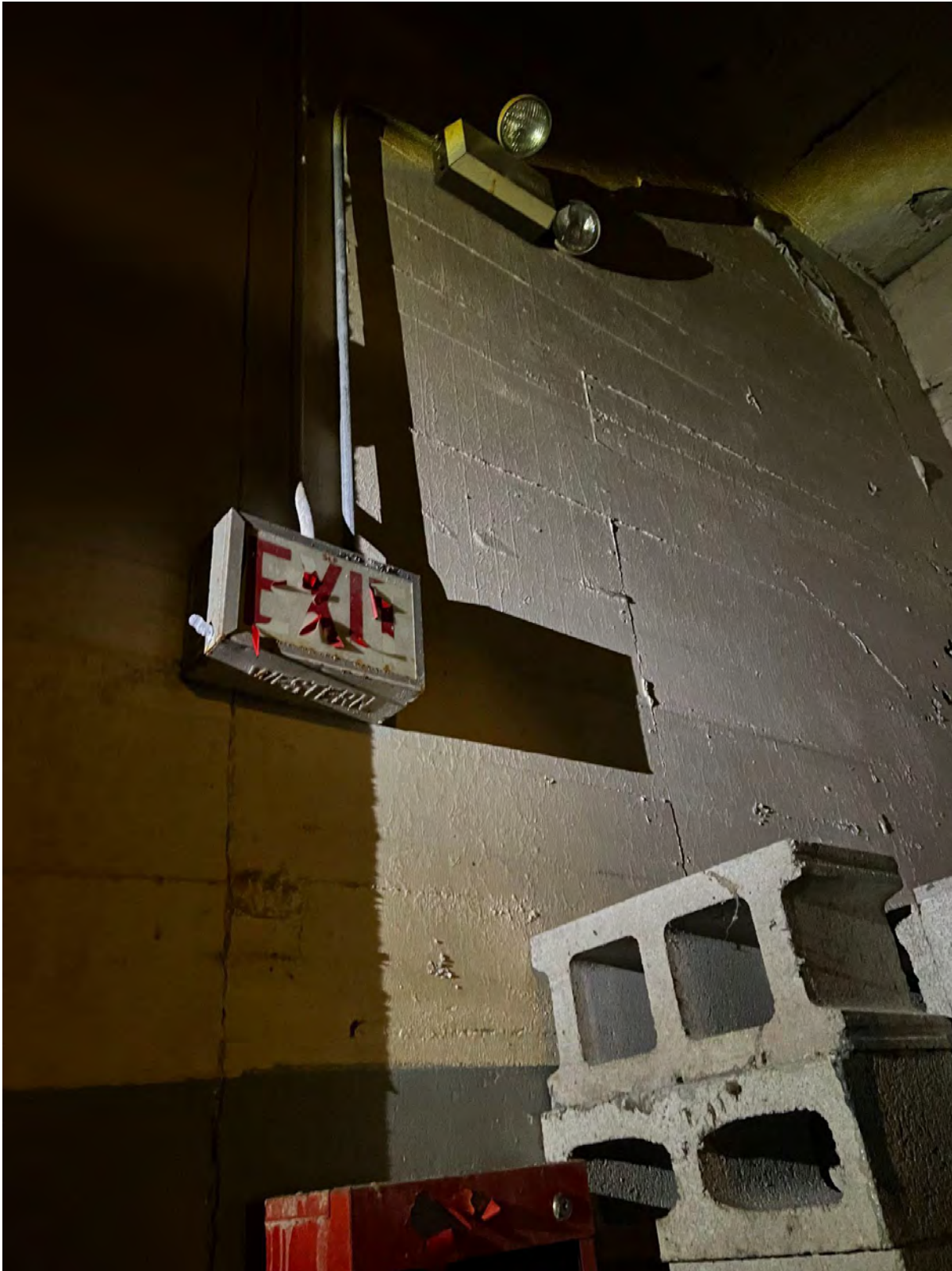
Basement: Damaged exit and emergency lights.
