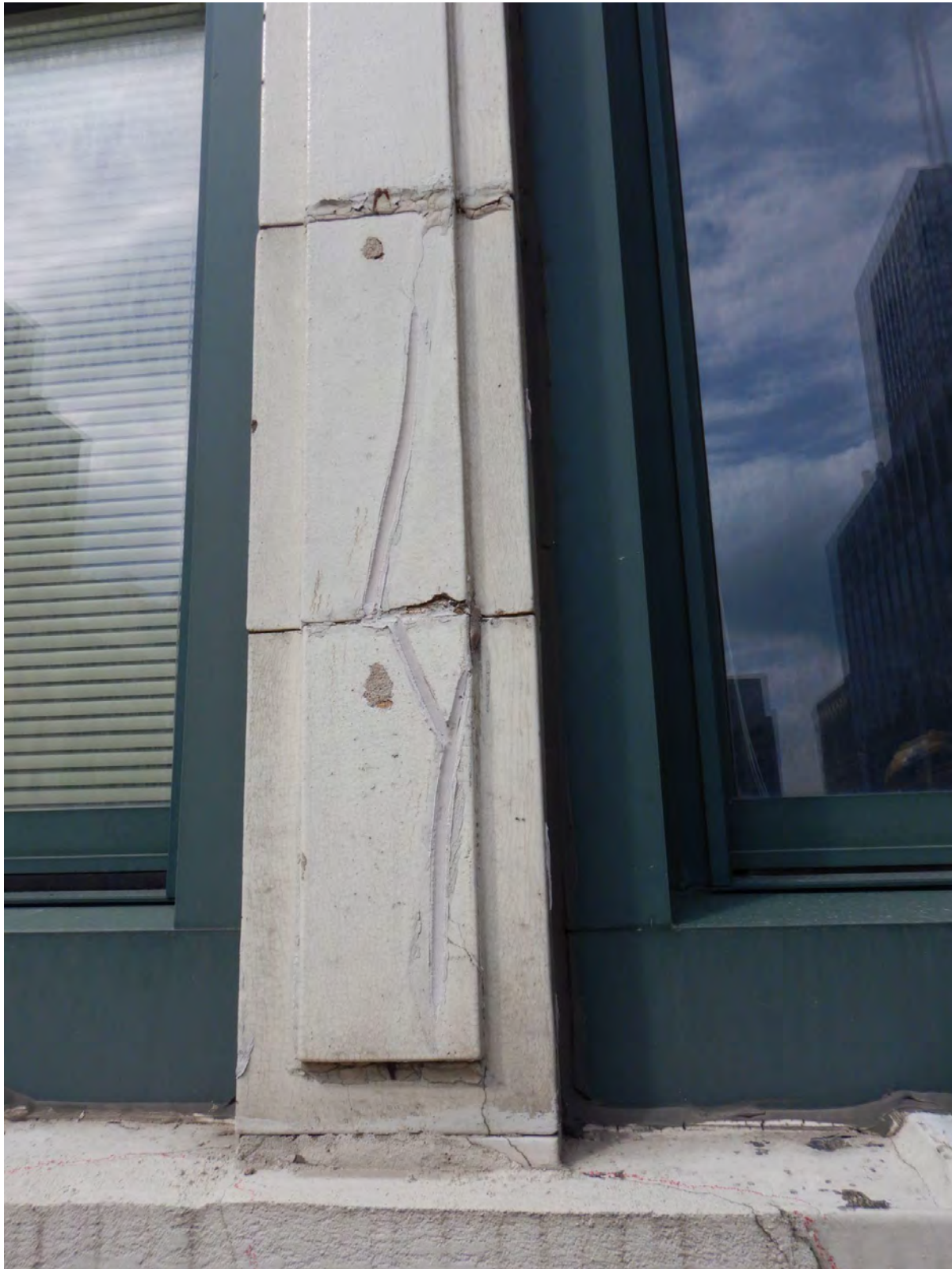
Overview of terra cotta mullion with previous repair efforts and newer crack
