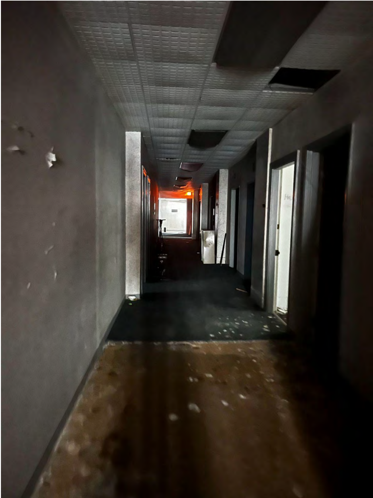
Upper Floor: Lights and electrical in corridor in poor shape
