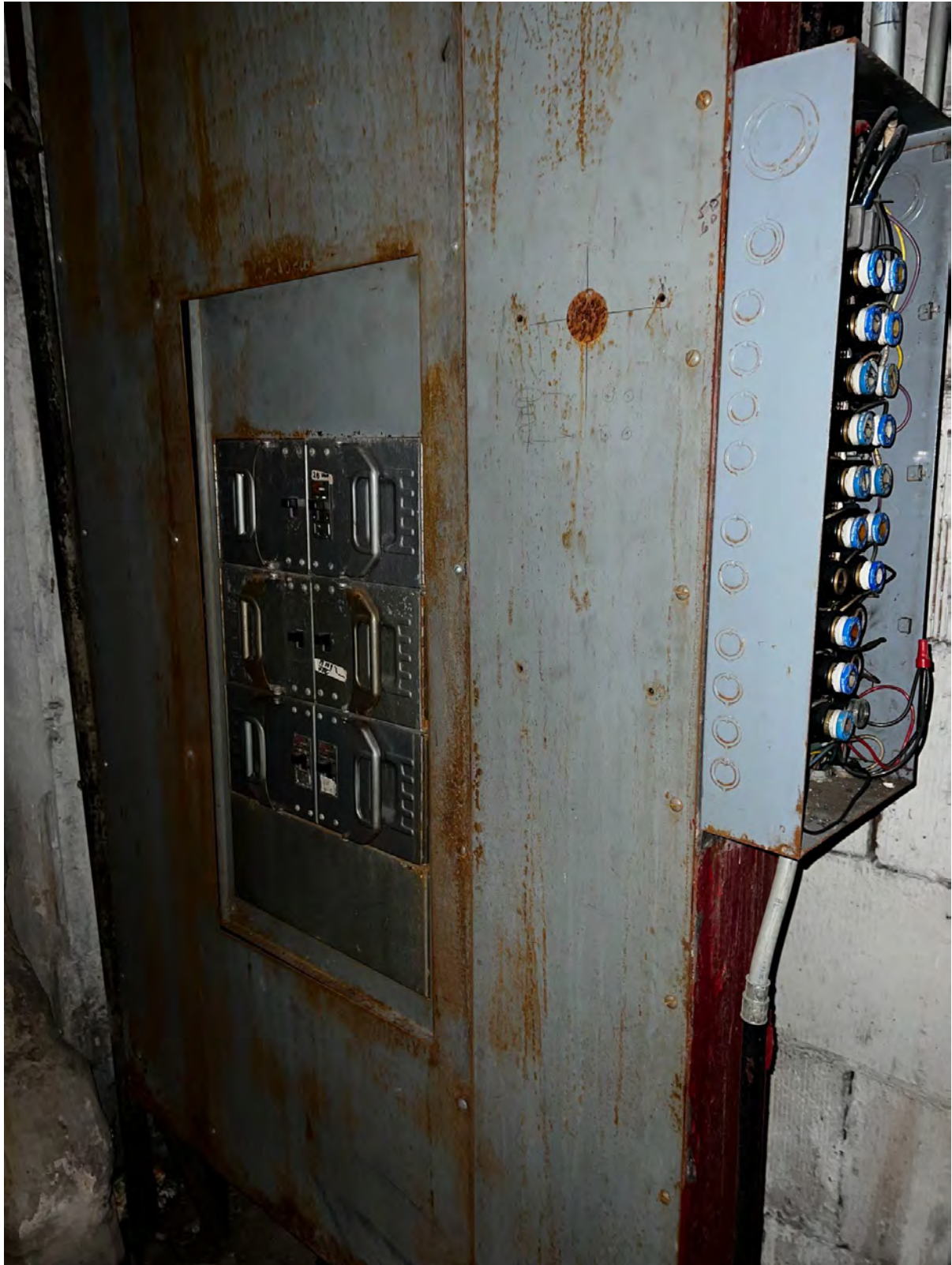
Sub-basement: Outdated panelboard with corrosion on exterior and missing covers.
