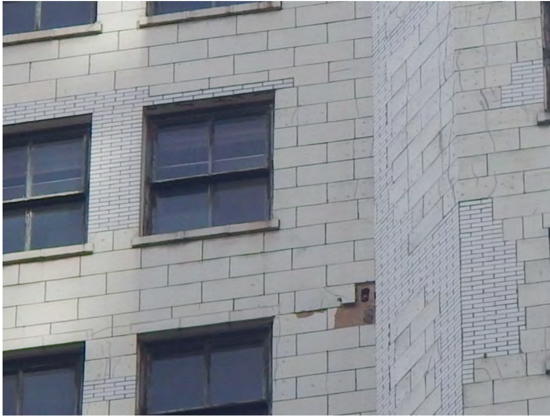
Overview of north elevation with terra cotta spalled units and cracked units
