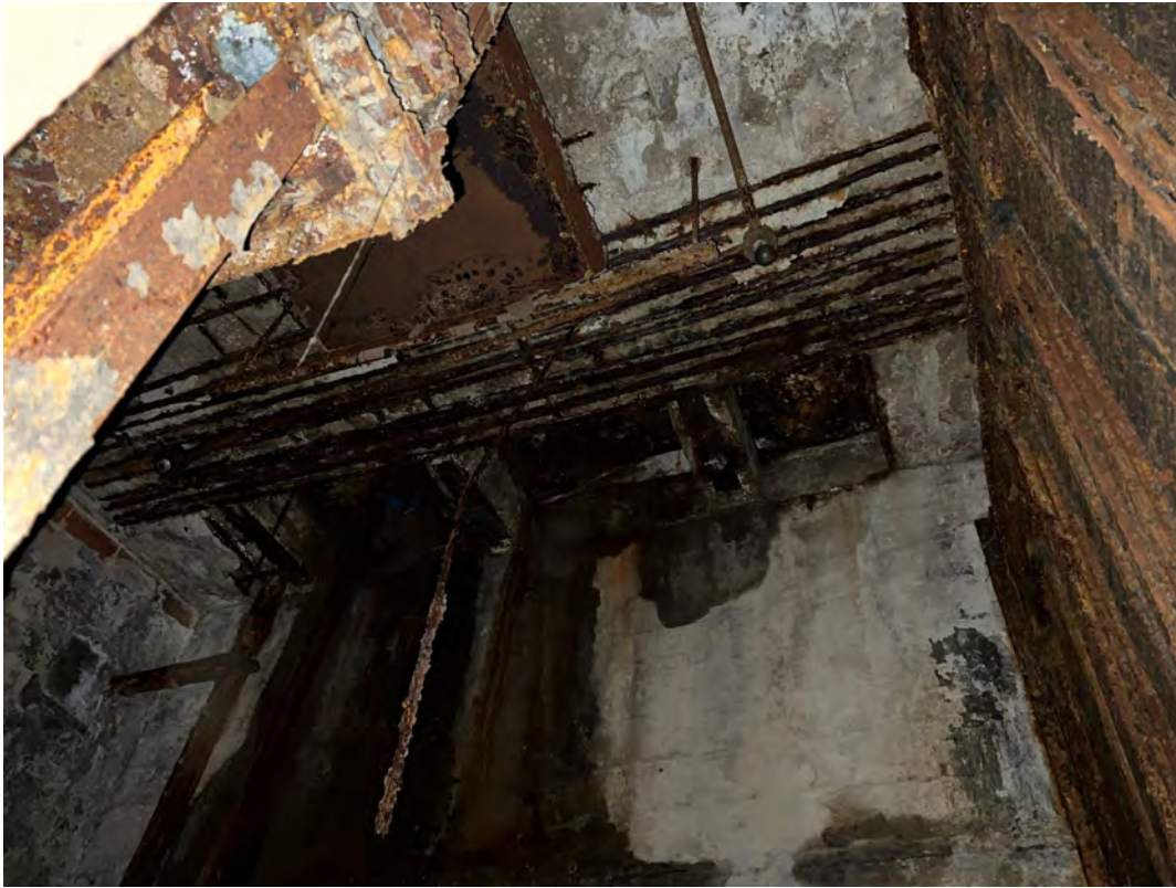
Middle basement slab from below: Southwest room heavily spalled and rebar is corroded
