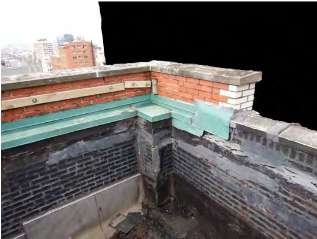
Southwest parapet corner with multiple copings, flashings, and temporary repairs
