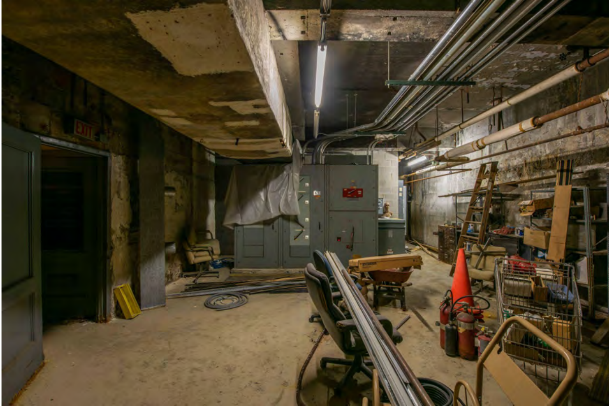
Lower Level 1 Switchgear
