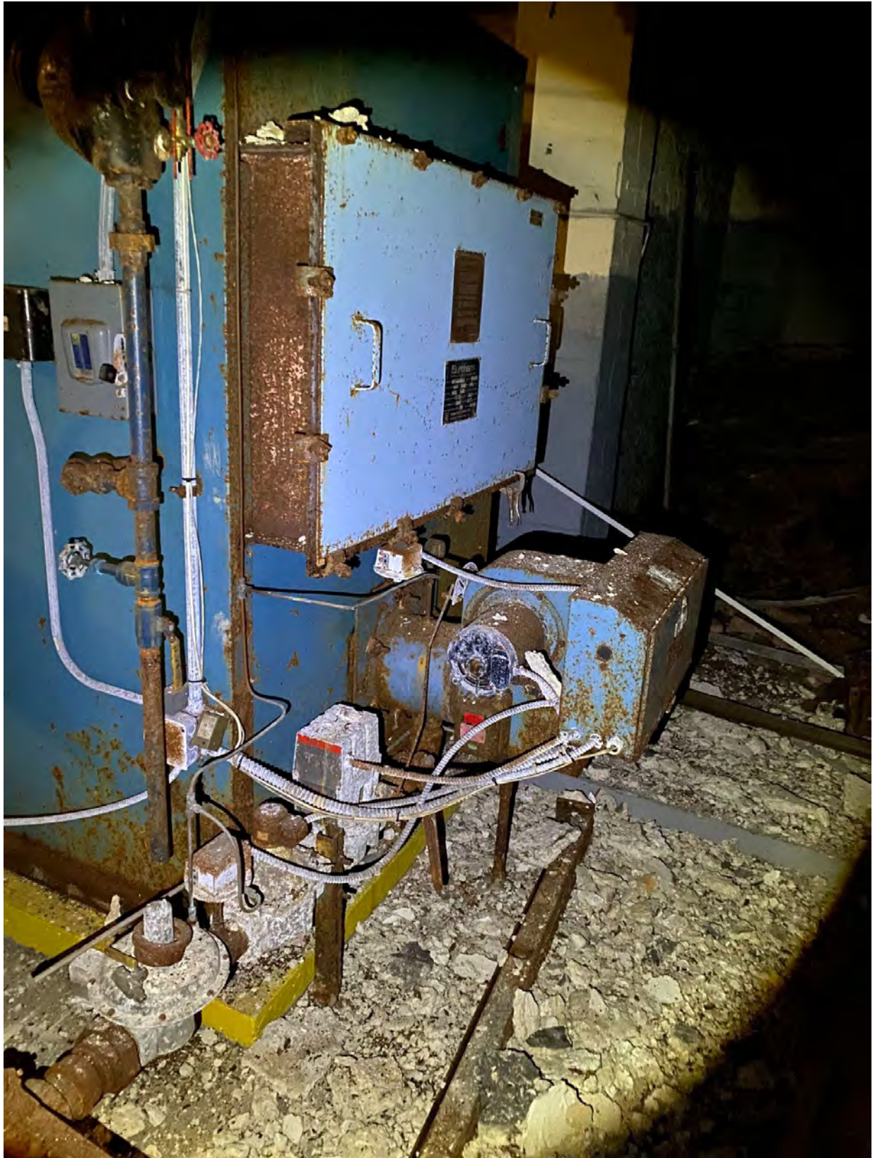
Basement 3 - Existing Steam Boiler
