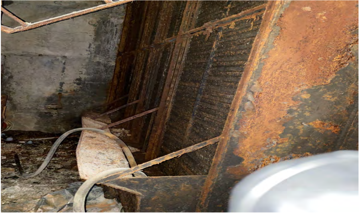
Basement 2 - Existing Outdoor air intake filter
