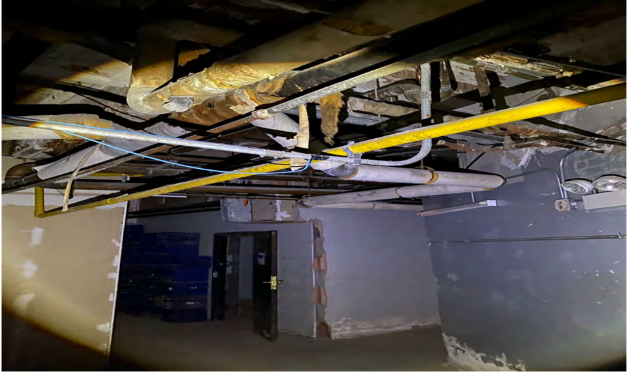
Basement 1 - Existing piping
