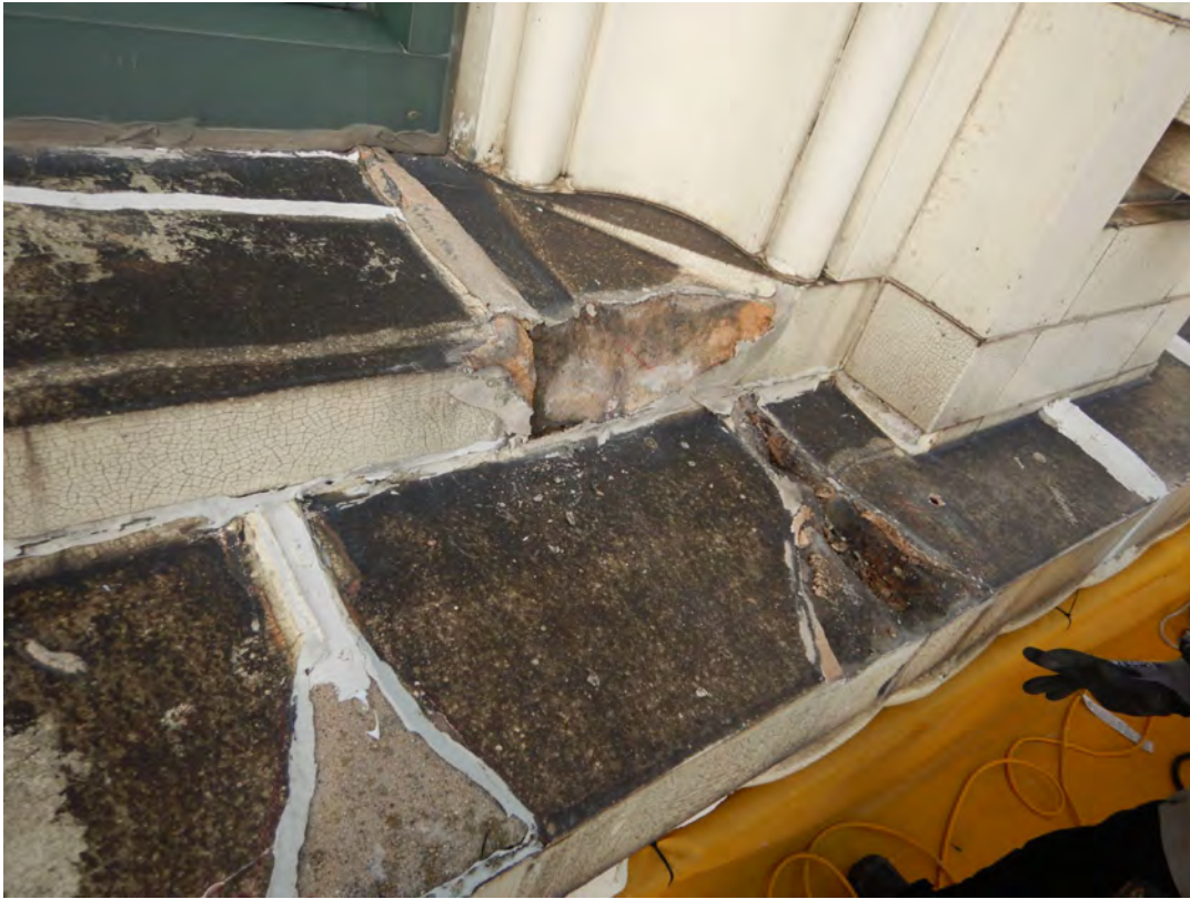
Overview of previous repair efforts and open joint at top of water table
