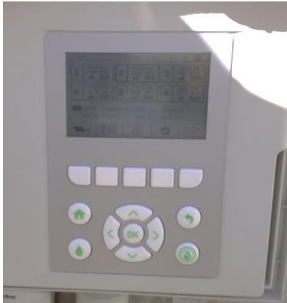
Figure 8. Photo of Control Box for Controller 1 Area
