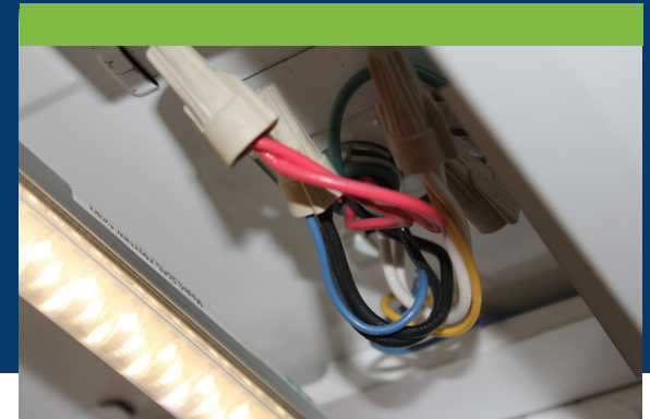
Ballast is disconnected. Sockets are wired directly to the branch circuit and provide line voltage. Photo credit Michael Myer, PNNL
