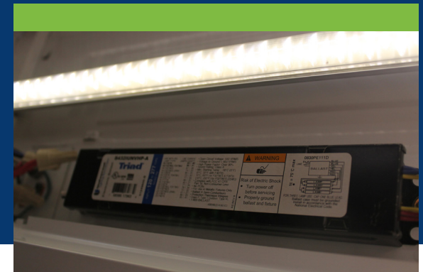
Type A TLED installed in the luminaire using the existing ballast. Photo credit Michael Myer, PNNL
