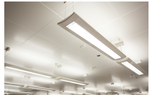
Linear pendants have both an uplight and downlight and can be challenging to retrofit to LED lighting. New fixtures are best.
