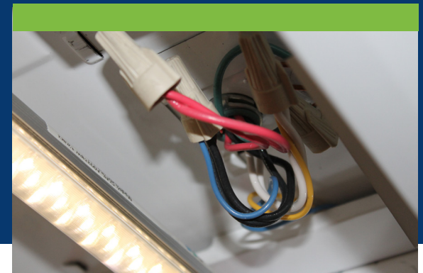
Ballast is disconnected. Sockets are wired directly to the branch circuit and provide line voltage.
