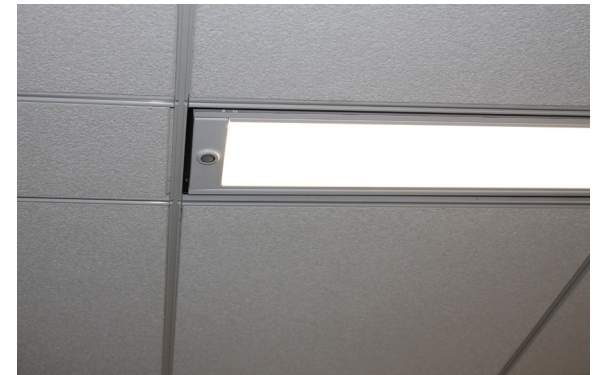
Troffer with embedded occupancy sensor
