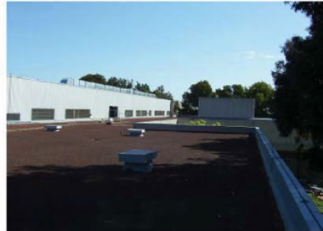
Example of a building that has no attic space. This is a roof with a mechanical penthouse.
