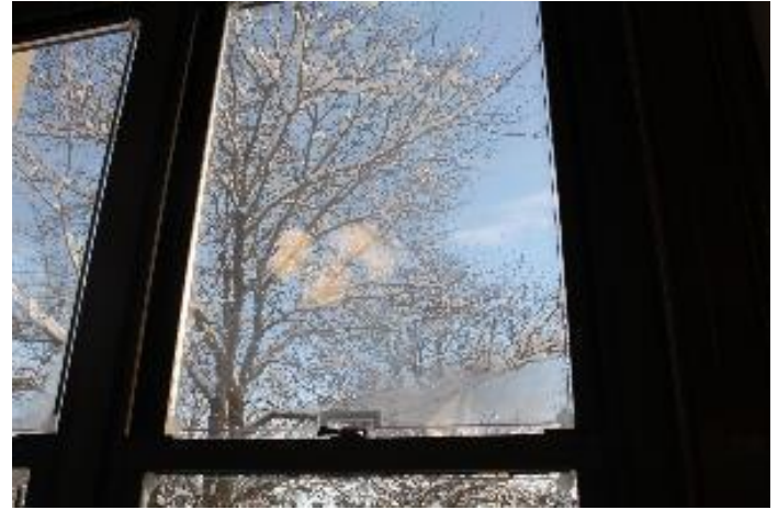
Condensation is between the panes of glass of the original window, indicating that the seal has failed.
