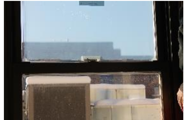
White border was a 3D-printed portion of a panel that surrounds the window lock (May 1, 2023).
