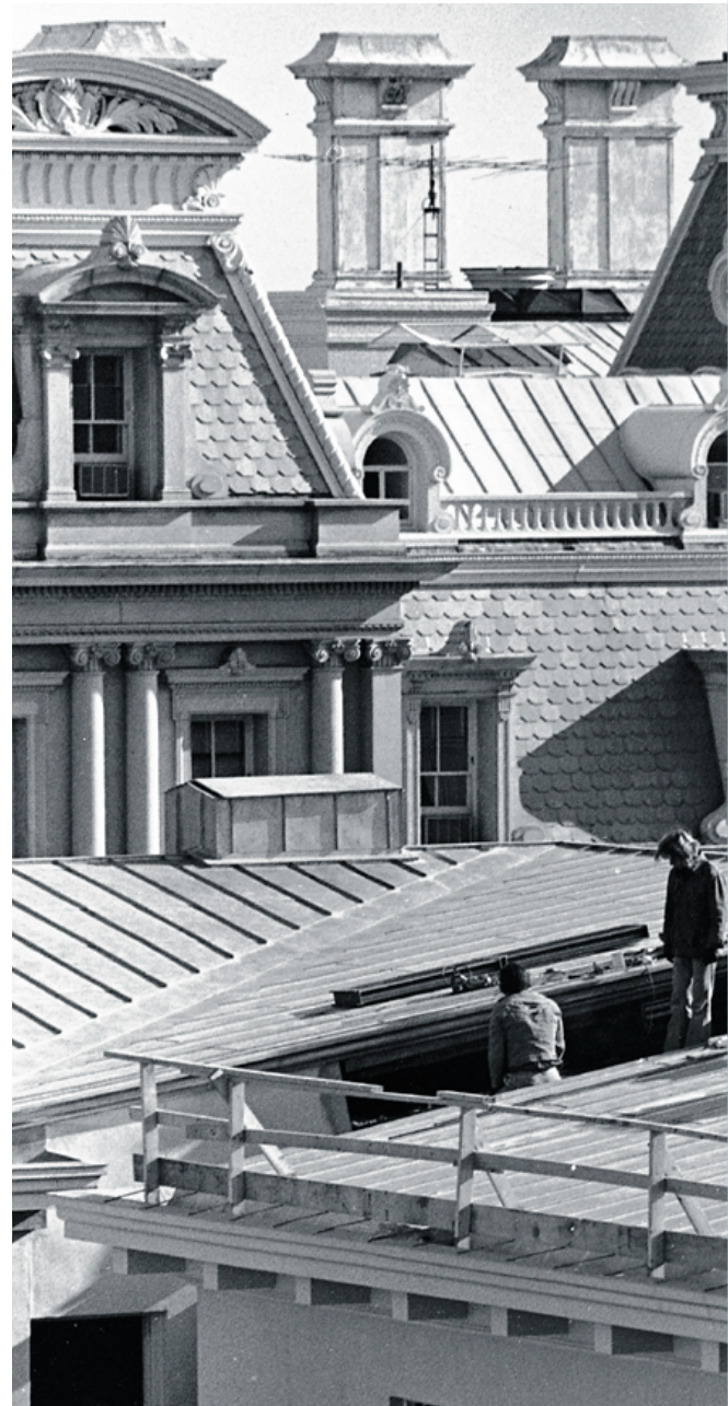
Workmen on the roof of the Winder Building, Washington, D.C. install a window as part of a renovation project.
