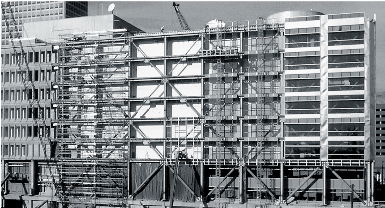
The W.F. Bennett Federal Building in Salt Lake City is the first federal building to use buckling-restrained brace technology.
