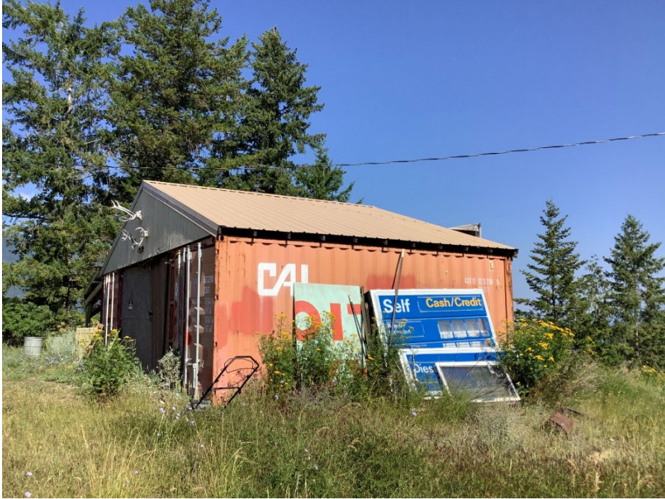
589 Figure 14. Oblique view of larger shed on the eastern side of the property. Oblique view of southern and 590 western facing façades, view toward northeast.
