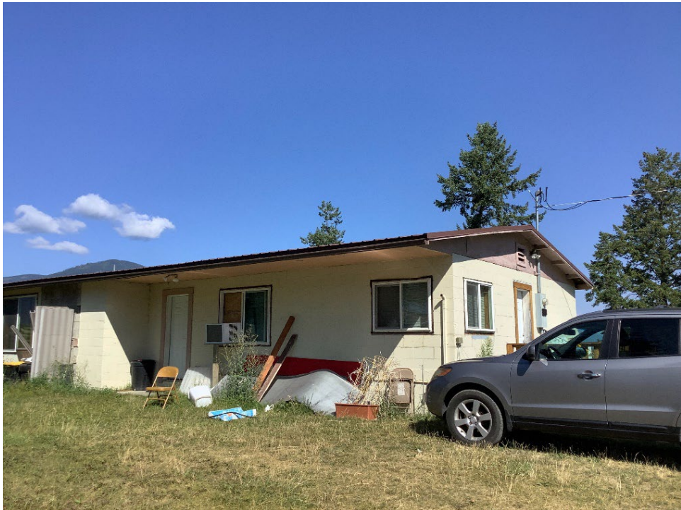
527 Figure 8. Detail of eaves, 147 Trading Post Road. Oblique view of south and east facing façades.
