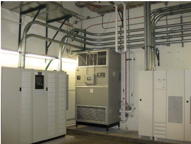
UPS room, two UPS and one CRAH units serving UPS room are shown
