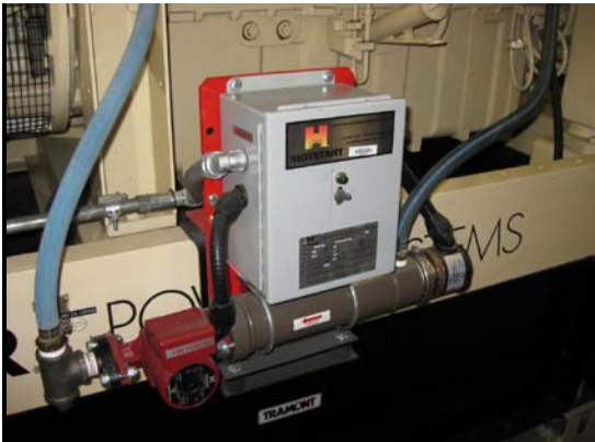
Generator Block heater pump and heater
