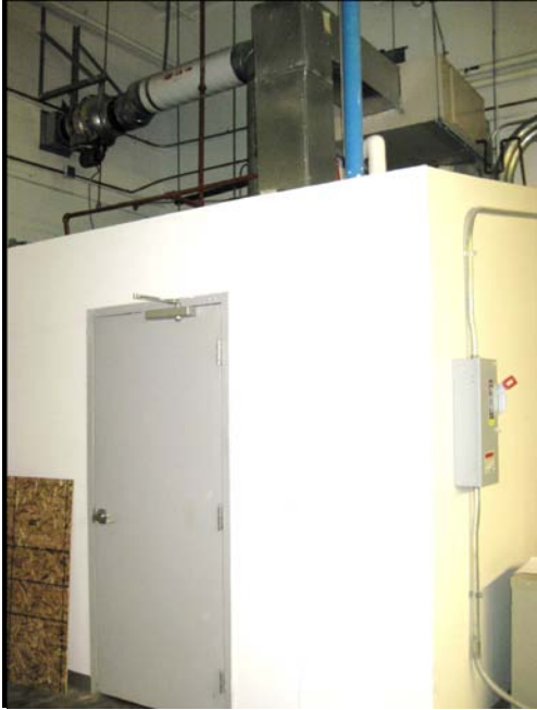
Battery room and its AC unit
