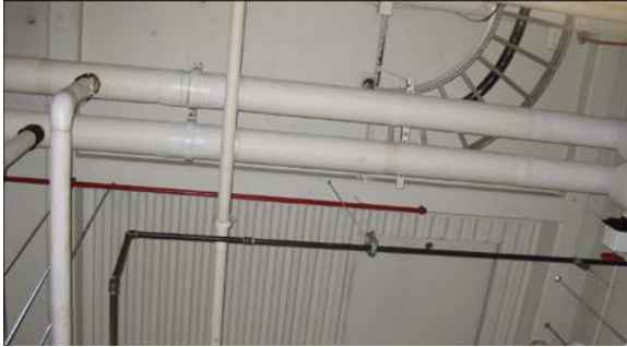
Chilled water pipes metering suggested location in AHU room adjacent to data center
