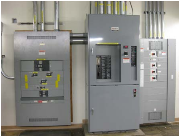
Panel DP-1-UPS in UPS room
