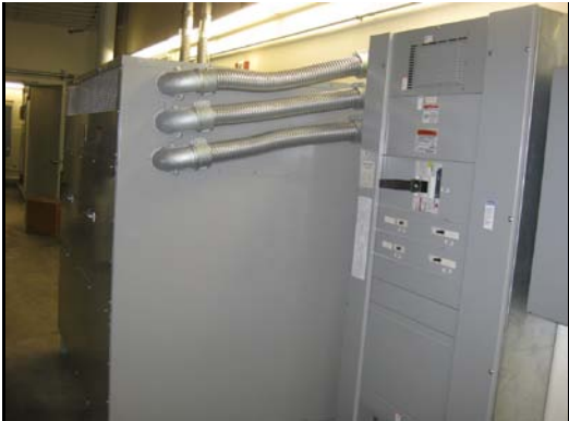
Panel DP-2-UPS in Air Handler room
