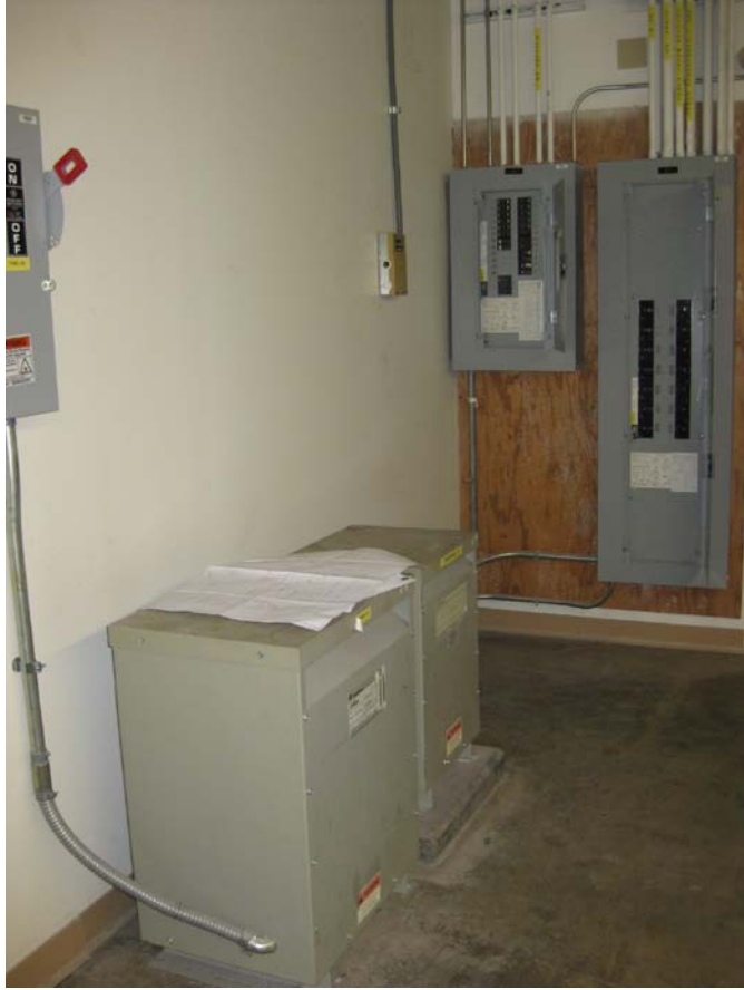
Panel B7A and related transformers in Air Handler room
